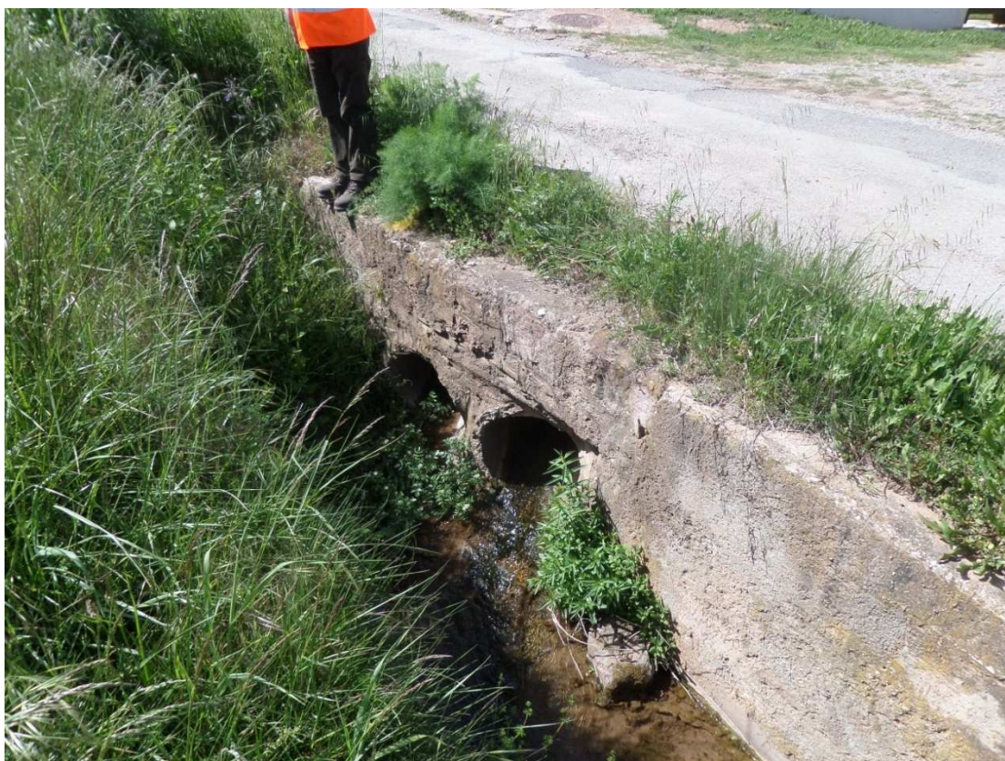
P40 : amont (Buse DN800) / aval (2 buses DN500)
