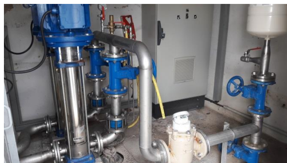
Station de pompage
