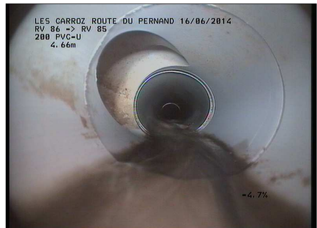
Photo: 22_4A, MPEG #: 160614_1, 00:00:53 5m, Raccordement correct à 10 h.
