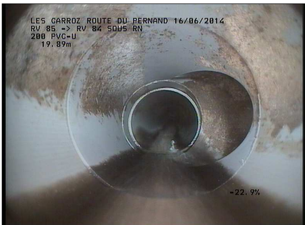
Photo: 23_4A, MPEG #: 160614_1, 00:01:37 20,27m, Raccordement correct à 03 h.
