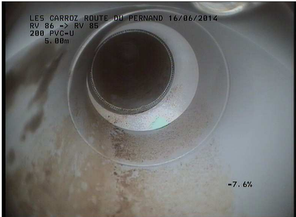
Photo: 22_4B, MPEG #: 160614_1, 00:00:53 5m, Raccordement correct à 10 h.
