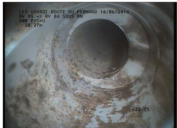
Photo: 23_4B, MPEG #: 160614_1, 00:01:37 20,27m, Raccordement correct à 03 h.
