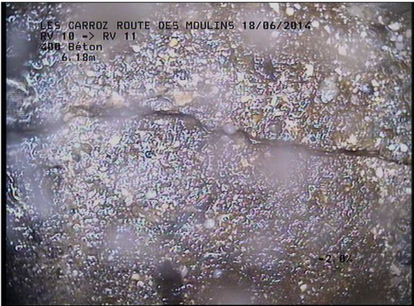
Photo: 10_3B, MPEG #: 180614_1, 00:00:51 6,18m, Fissure transversale (circulaire)
