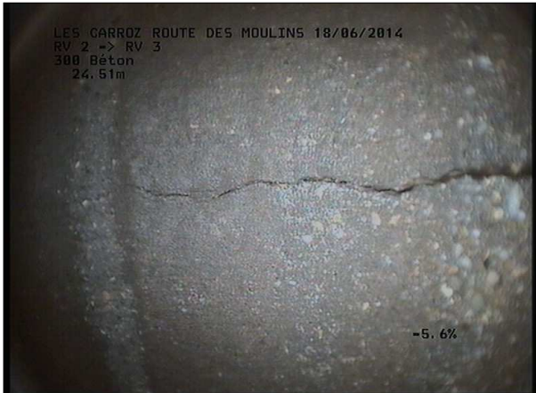
Photo: 2_7B, MPEG #: 180614_1, 00:03:01 24,51m, Fissure transversale (circulaire)
