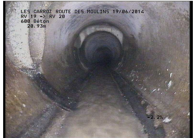
Photo: 19_3A, MPEG #: 180614_1, 00:01:23 22,06m, Raccordement direct à 09 h.
