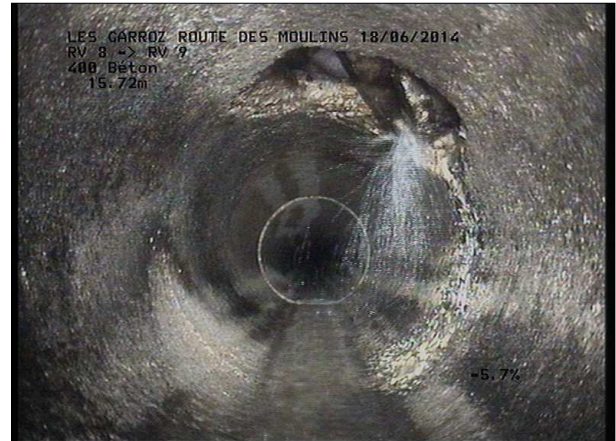
Photo: 8_6A, MPEG #: 180614_1, 00:02:52 16,25m, Raccordement direct à 01 h.
