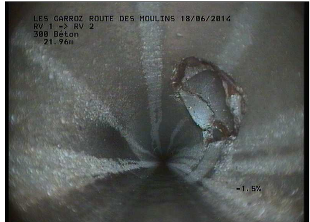
Photo: 1_11A, MPEG #: 180614_1, 00:04:18 22,48m, Raccordement direct à 02 h.
