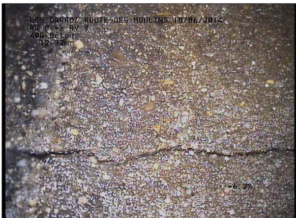
Photo: 8_4B, MPEG #: 180614_1, 00:01:36 12,32m, Fissure transversale (circulaire)
