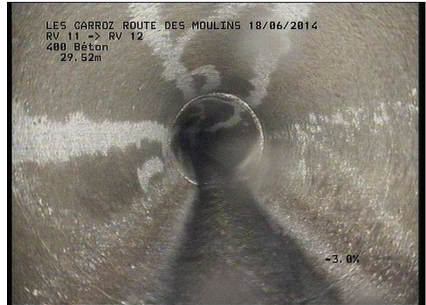
Photo: 11_8A, MPEG #: 180614_1, 00:04:36 29,9m, Fissure transversale (circulaire)
