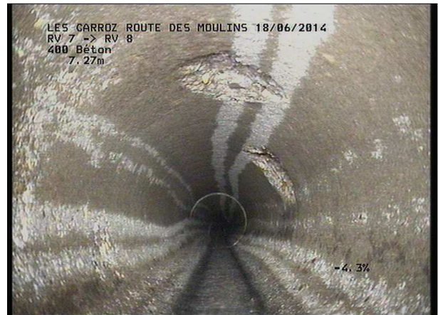
Photo: 7_2A, MPEG #: 180614_1, 00:00:39 7,81m, Perforation à 12 h.
