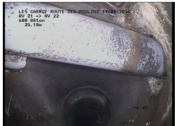
Photo: 21_5A, MPEG #: 180614_1, 00:02:26 25,93m, Raccordement direct à 09 h.
