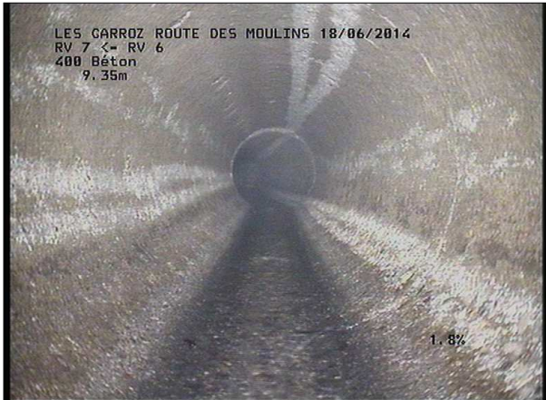
Photo: 6_4A, MPEG #: 180614_1, 00:01:36 9,88m, Fissure transversale (circulaire)
