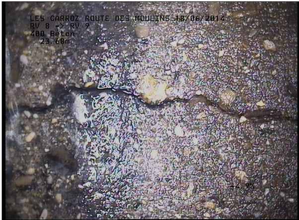
Photo: 8_9B, MPEG #: 180614_1, 00:04:21 23,68m, Fissure transversale (circulaire)
