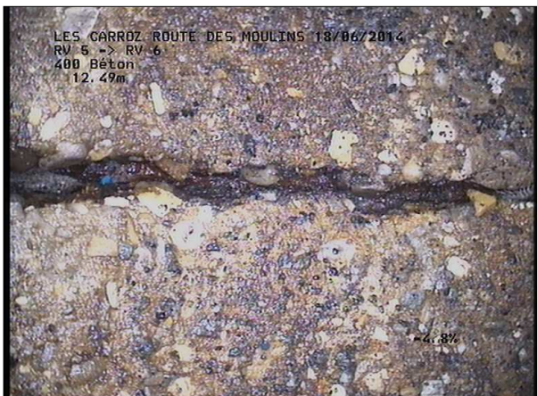
Photo: 5_2B, MPEG #: 180614_1, 00:01:00 12,49m, Fissure transversale (circulaire)
