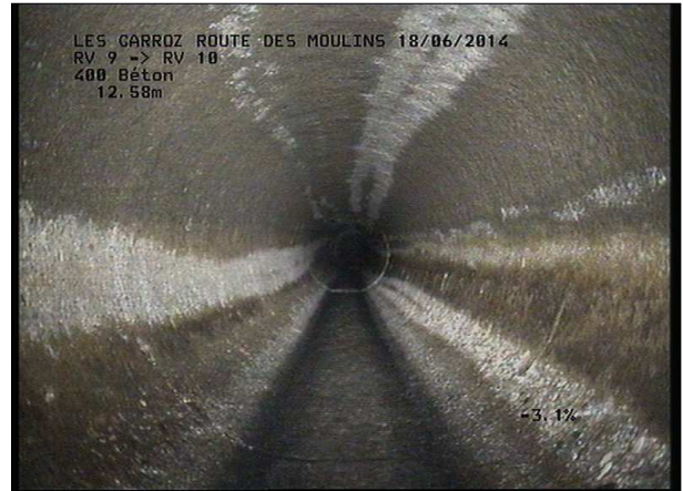
Photo: 9_2A, MPEG #: 180614_1, 00:01:11 13,09m, Fissure transversale (circulaire)
