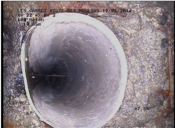
Photo: 22_3B, MPEG #: 180614_1, 00:00:55 10,35m, Raccordement direct à 09 h.
