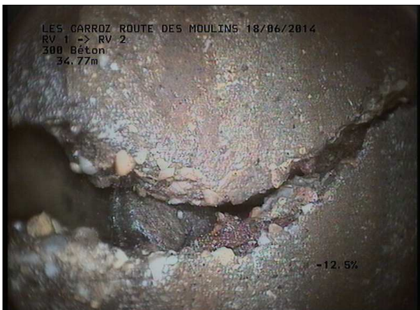
Photo: 1_15B, MPEG #: 180614_1, 00:06:07 34,77m, Fissure transversale (circulaire)
