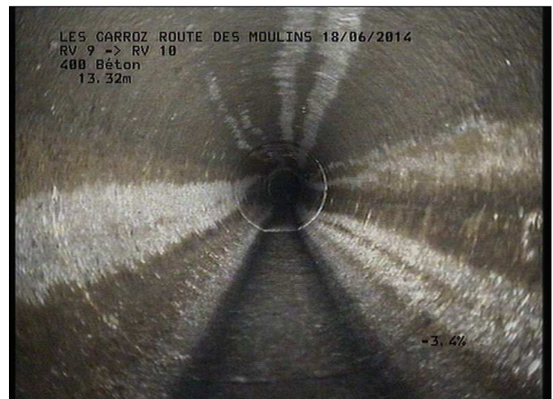
Photo: 9_3A, MPEG #: 180614_1, 00:01:35 13,77m, Fissure transversale (circulaire)
