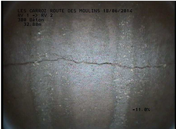
Photo: 1_14B, MPEG #: 180614_1, 00:05:43 32,88m, Fissure transversale (circulaire)
