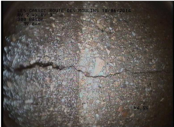
Photo: 2_9B, MPEG #: 180614_1, 00:04:34 39,64m, Fissure transversale (circulaire)
