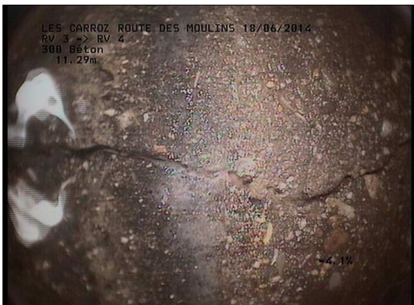
Photo: 3_6B, MPEG #: 180614_1, 00:02:11 11,29m, Fissure transversale (circulaire)
