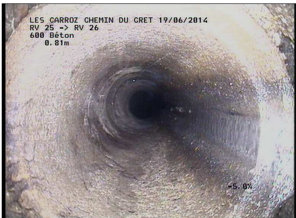
Photo: 25_2B, MPEG #: 180614_1, 00:00:07 0,81m, Raccordement direct à 03 h.
