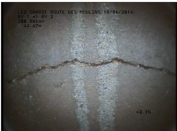
Photo: 1_17B, MPEG #: 180614_1, 00:07:19 44,47m, Fissure transversale (circulaire)
