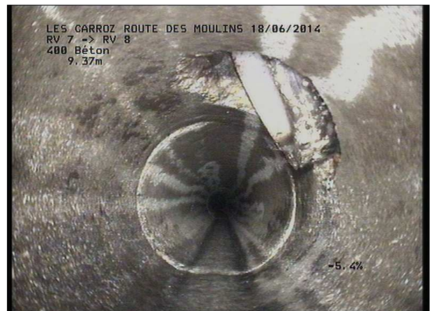
Photo: 7_5A, MPEG #: 180614_1, 00:01:58 9,37m, Raccordement direct à 01 h.
