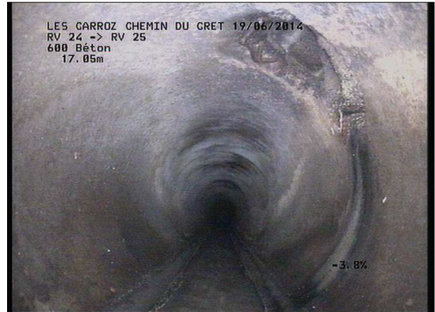
Photo: 24_4A, MPEG #: 180614_1, 00:01:53 18,11m, Raccordement direct à 01 h.
