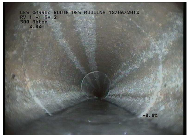
Photo: 1_3A, MPEG #: 180614_1, 00:00:52 5,05m, Fissure transversale (circulaire)
