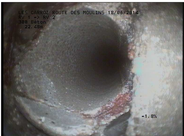
Photo: 1_11B, MPEG #: 180614_1, 00:04:18 22,48m, Raccordement direct à 02 h.
