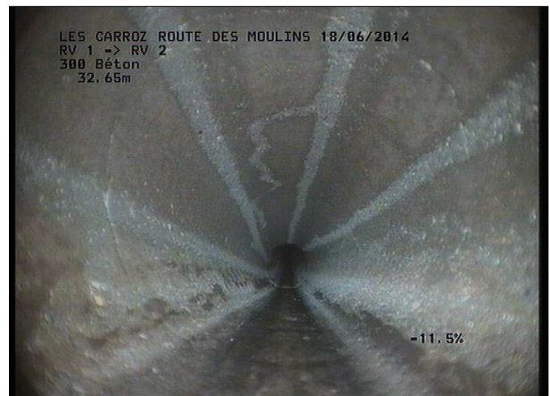
Photo: 1_14A, MPEG #: 180614_1, 00:05:43 32,88m, Fissure transversale (circulaire)
