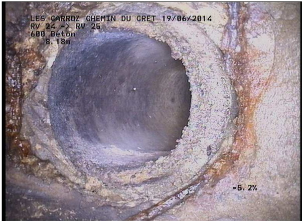
Photo: 24_3B, MPEG #: 180614_1, 00:01:02 8,18m, Raccordement direct à 01 h.
