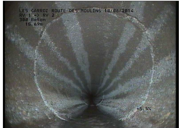
Photo: 1_9A, MPEG #: 180614_1, 00:03:14 16m, Fissure transversale (circulaire)
