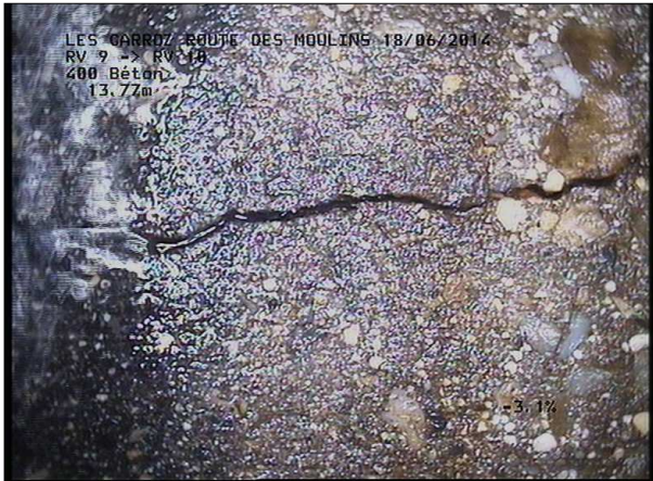
Photo: 9_3B, MPEG #: 180614_1, 00:01:35 13,77m, Fissure transversale (circulaire)
