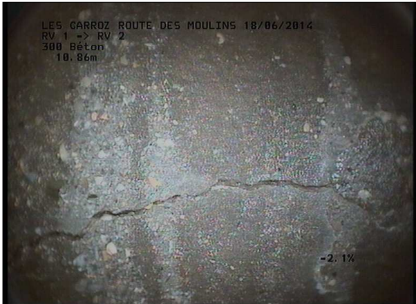
Photo: 1_8B, MPEG #: 180614_1, 00:02:34 10,86m, Fissure transversale (circulaire)
