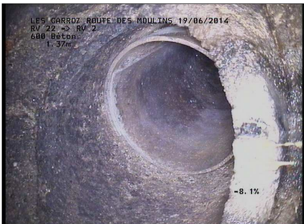
Photo: 22_2B, MPEG #: 180614_1, 00:00:05 1,37m, Raccordement direct à 02 h.
