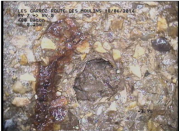
Photo: 7_2B, MPEG #: 180614_1, 00:00:44 8,25m, Perforation à 02 h.
