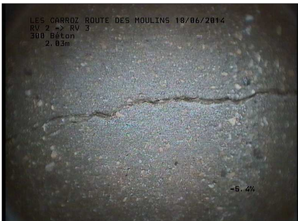
Photo: 2_2B, MPEG #: 180614_1, 00:00:14 2,03m, Fissure transversale (circulaire)
