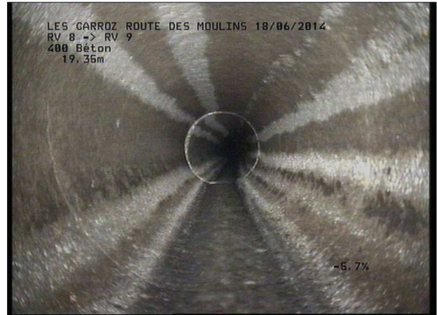
Photo: 8_8A, MPEG #: 180614_1, 00:03:47 19,79m, Fissure transversale (circulaire)
