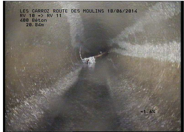
Photo: 10_4A, MPEG #: 180614_1, 00:02:33 21,37m, Fissure transversale fermée (circulaire)
