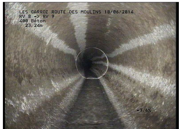
Photo: 8_9A, MPEG #: 180614_1, 00:04:21 23,68m, Fissure transversale (circulaire)
