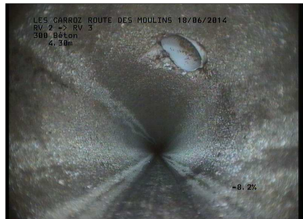
Photo: 2_3A, MPEG #: 180614_1, 00:00:44 4,65m, Raccordement direct à 01 h.
