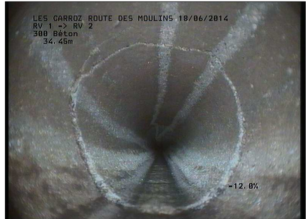
Photo: 1_15A, MPEG #: 180614_1, 00:06:07 34,77m, Fissure transversale (circulaire)
