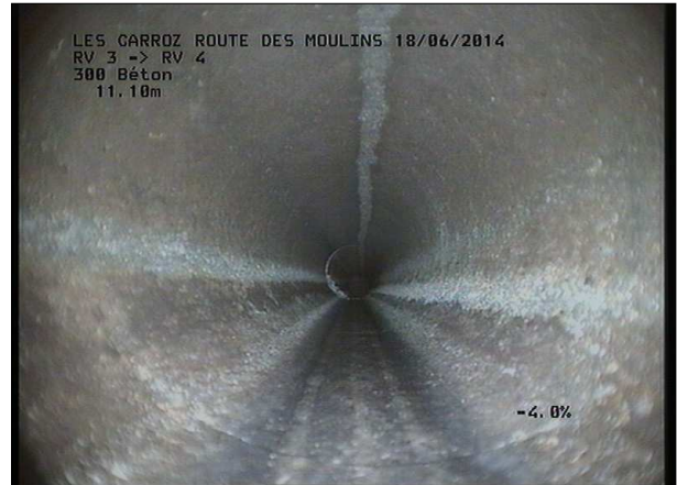
Photo: 3_6A, MPEG #: 180614_1, 00:02:11 11,29m, Fissure transversale (circulaire)
