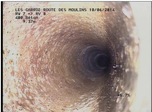
Photo: 7_5B, MPEG #: 180614_1, 00:01:58 9,37m, Raccordement direct à 01 h.
