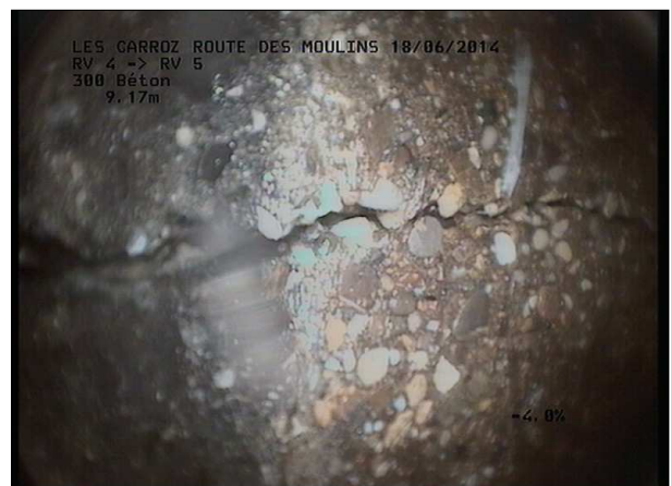
Photo: 4_5B, MPEG #: 180614_1, 00:01:31 9,17m, Fissure transversale (circulaire)
