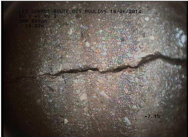
Photo: 1_10B, MPEG #: 180614_1, 00:03:44 18,82m, Fissure transversale (circulaire)
