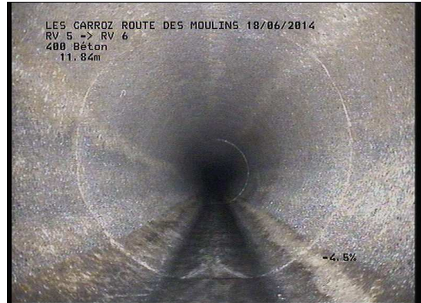
Photo: 5_2A, MPEG #: 180614_1, 00:01:00 12,49m, Fissure transversale (circulaire)
