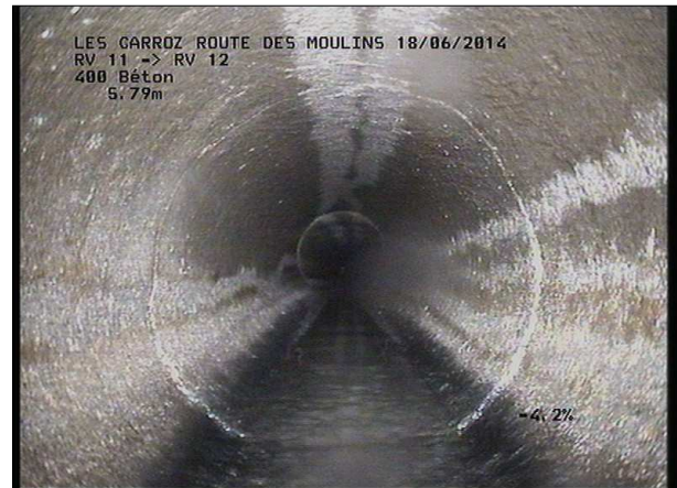
Photo: 11_2A, MPEG #: 180614_1, 00:00:40 6,38m, Fissure transversale (circulaire)
