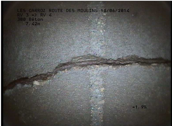
Photo: 3_5B, MPEG #: 180614_1, 00:01:41 7,42m, Fissure transversale (circulaire)
