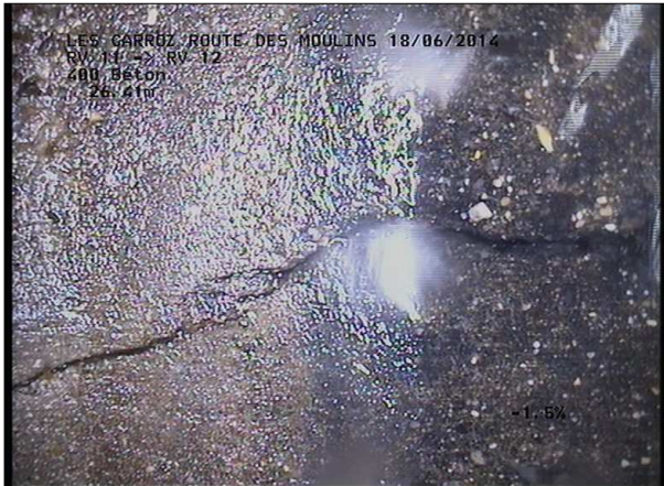
Photo: 11_7B, MPEG #: 180614_1, 00:03:56 26,41m, Fissure transversale (circulaire)
