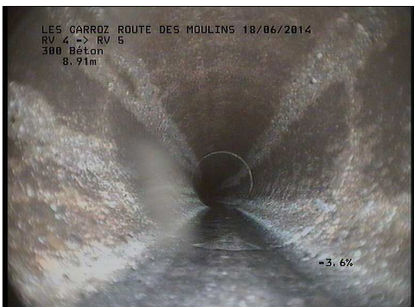
Photo: 4_5A, MPEG #: 180614_1, 00:01:31 9,17m, Fissure transversale (circulaire)
