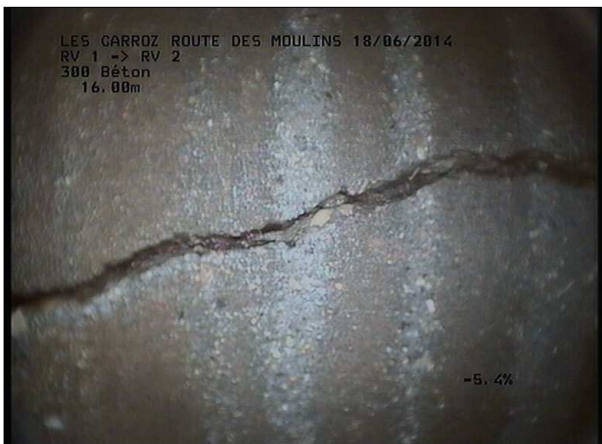
Photo: 1_9B, MPEG #: 180614_1, 00:03:14 16m, Fissure transversale (circulaire)
