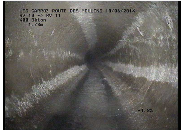
Photo: 10_2A, MPEG #: 180614_1, 00:00:14 2,26m, Fissure transversale (circulaire)
