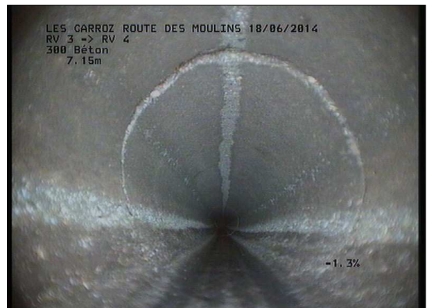
Photo: 3_5A, MPEG #: 180614_1, 00:01:41 7,42m, Fissure transversale (circulaire)
