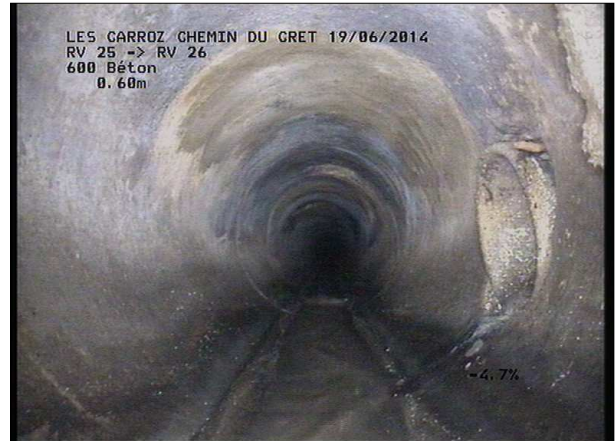
Photo: 25_2A, MPEG #: 180614_1, 00:00:07 0,81m, Raccordement direct à 03 h.
