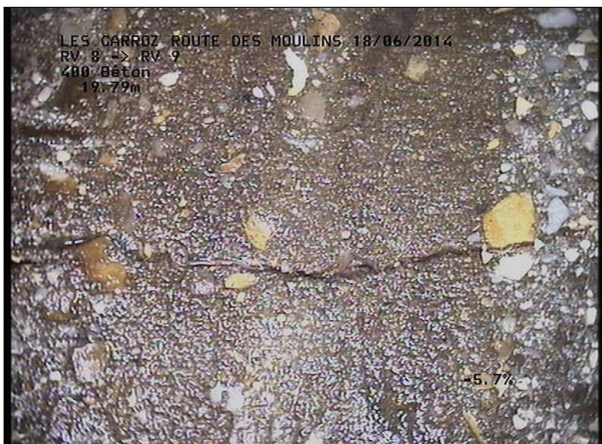
Photo: 8_8B, MPEG #: 180614_1, 00:03:47 19,79m, Fissure transversale (circulaire)
