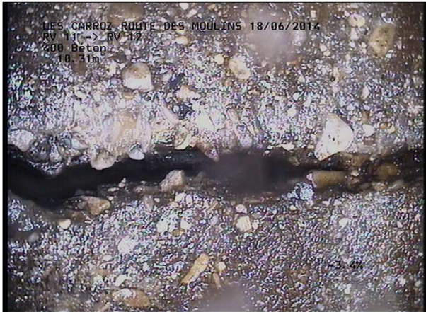
Photo: 11_3B, MPEG #: 180614_1, 00:01:18 10,31m, Fissure transversale (circulaire)
