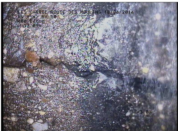
Photo: 9_2B, MPEG #: 180614_1, 00:01:11 13,09m, Fissure transversale (circulaire)
