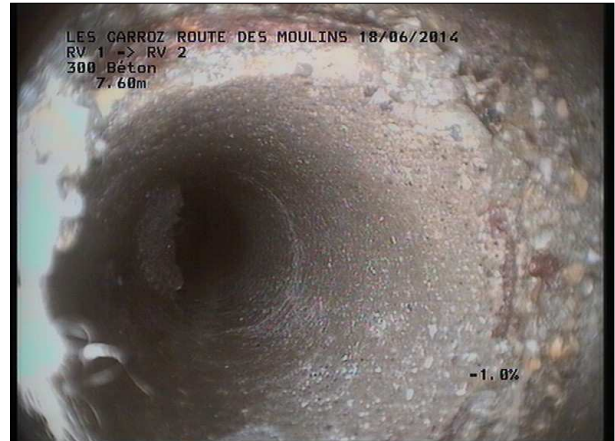
Photo: 1_6B, MPEG #: 180614_1, 00:01:51 7,6m, Raccordement direct à 09 h.
