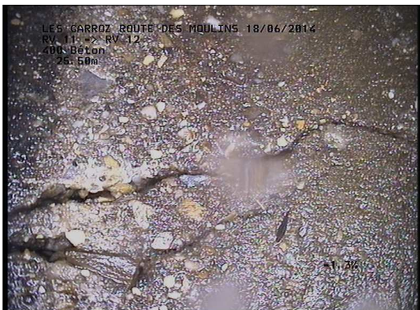
Photo: 11_6B, MPEG #: 180614_1, 00:03:32 25,5m, Fissure transversale (circulaire)
