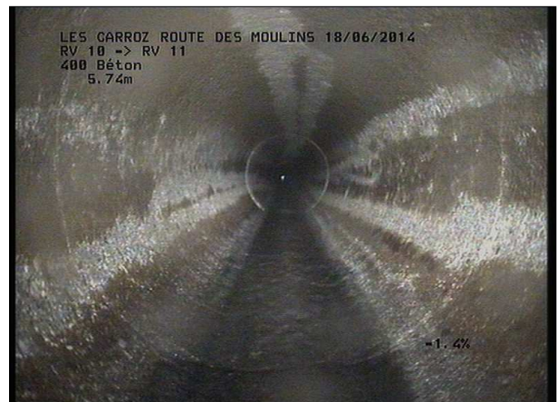
Photo: 10_3A, MPEG #: 180614_1, 00:00:51 6,18m, Fissure transversale (circulaire)
