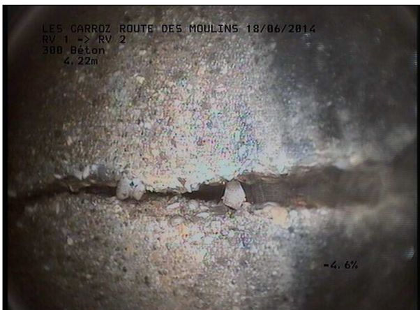
Photo: 1_2B, MPEG #: 180614_1, 00:00:30 4,22m, Fissure transversale (circulaire)
