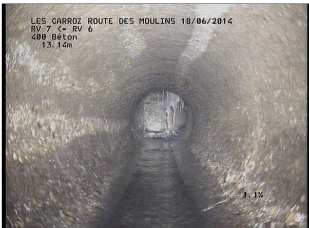
Photo: 6_5A, MPEG #: 180614_1, 00:02:44 13,64m, Fissure transversale (circulaire)
