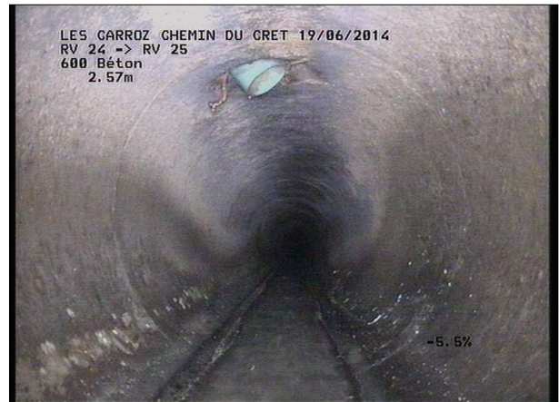
Photo: 24_2A, MPEG #: 180614_1, 00:00:13 3,99m, Raccordement direct à 11 h.
