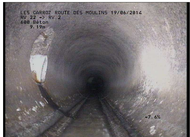
Photo: 22_3A, MPEG #: 180614_1, 00:00:55 10,35m, Raccordement direct à 09 h.
