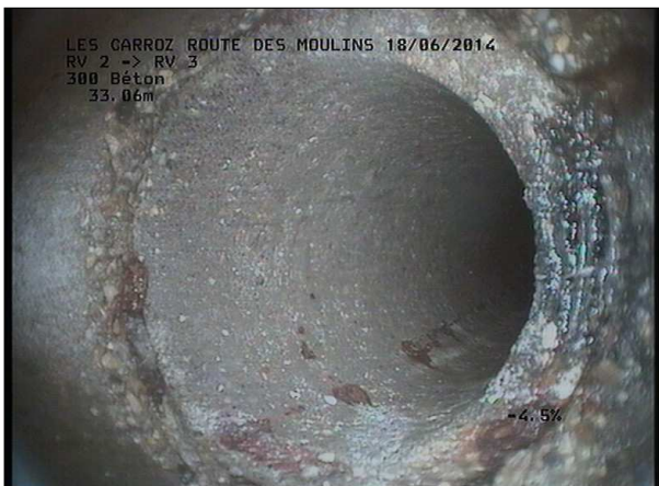
Photo: 2_8B, MPEG #: 180614_1, 00:03:52 33,06m, Raccordement direct à 02 h.
