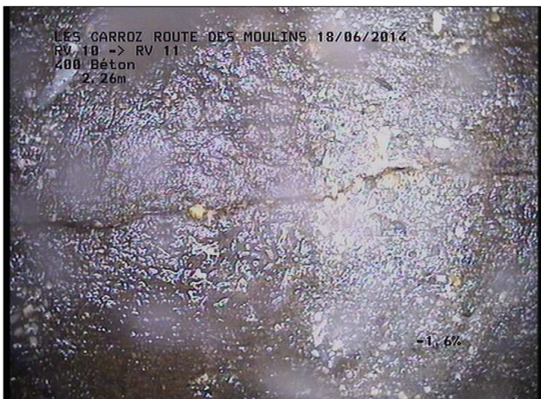
Photo: 10_2B, MPEG #: 180614_1, 00:00:14 2,26m, Fissure transversale (circulaire)
