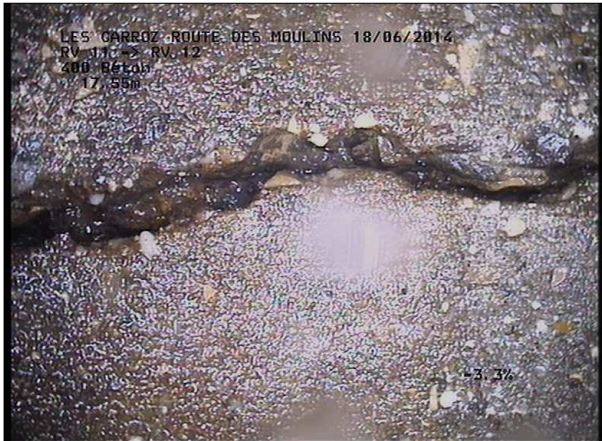
Photo: 11_5B, MPEG #: 180614_1, 00:02:29 17,55m, Fissure transversale (circulaire)
