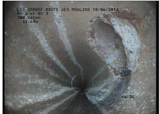
Photo: 2_8A, MPEG #: 180614_1, 00:03:52 33,06m, Raccordement direct à 02 h.
