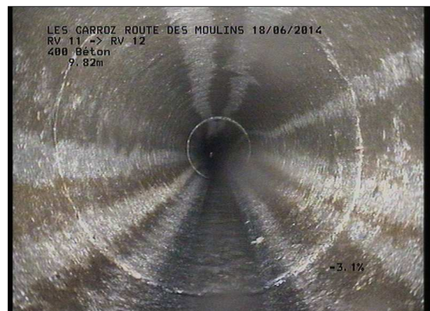
Photo: 11_3A, MPEG #: 180614_1, 00:01:18 10,31m, Fissure transversale (circulaire)
