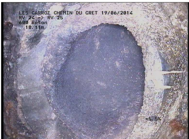
Photo: 24_4B, MPEG #: 180614_1, 00:01:53 18,11m, Raccordement direct à 01 h.
