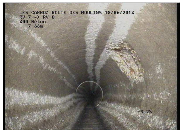
Photo: 7_3A, MPEG #: 180614_1, 00:00:44 8,25m, Perforation à 02 h.
