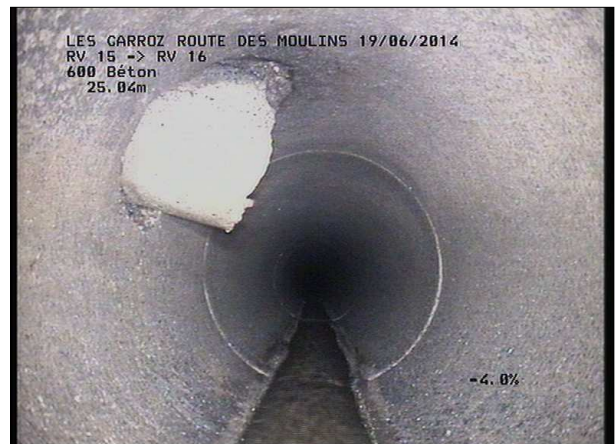
Photo: 15_3A, MPEG #: 180614_1, 00:02:05 26,25m, Raccordement direct à 11 h.
