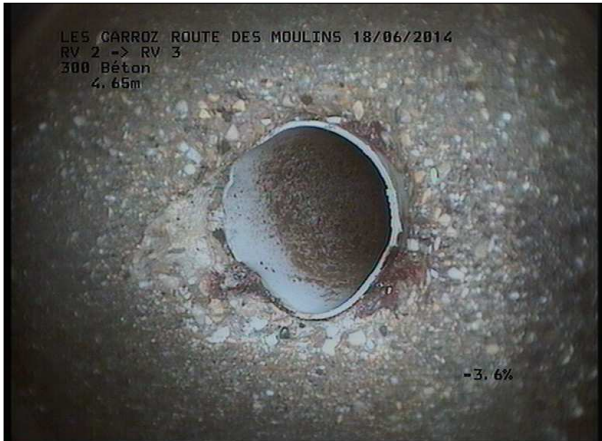
Photo: 2_3B, MPEG #: 180614_1, 00:00:44 4,65m, Raccordement direct à 01 h.
