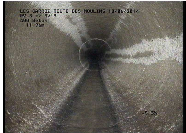
Photo: 8_4A, MPEG #: 180614_1, 00:01:36 12,32m, Fissure transversale (circulaire)
