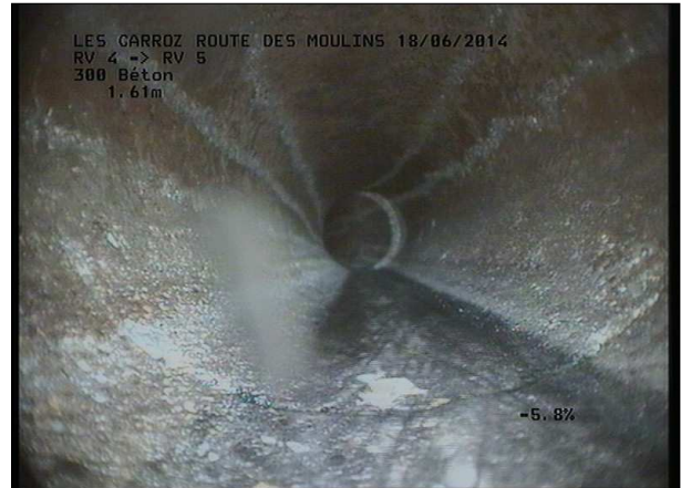
Photo: 4_2A, MPEG #: 180614_1, 00:00:16 1,78m, Fissure transversale (circulaire)
