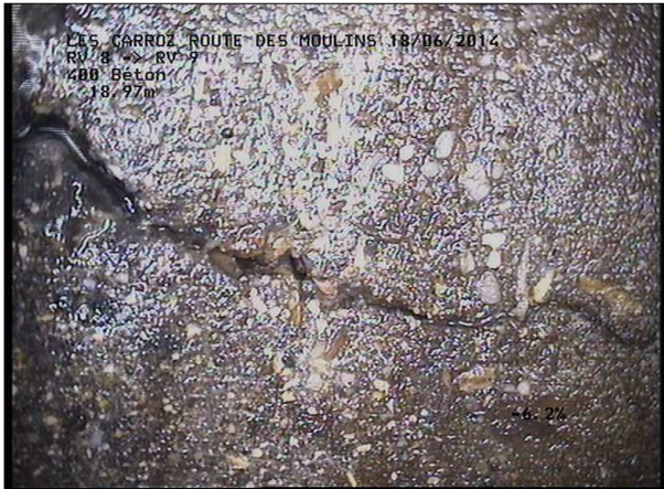
Photo: 8_7B, MPEG #: 180614_1, 00:03:22 18,97m, Fissure transversale (circulaire)
