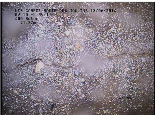
Photo: 10_4B, MPEG #: 180614_1, 00:02:33 21,37m, Fissure transversale fermée (circulaire)
