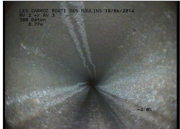
Photo: 2_4A, MPEG #: 180614_1, 00:01:13 9,01m, Fissure transversale (circulaire)
