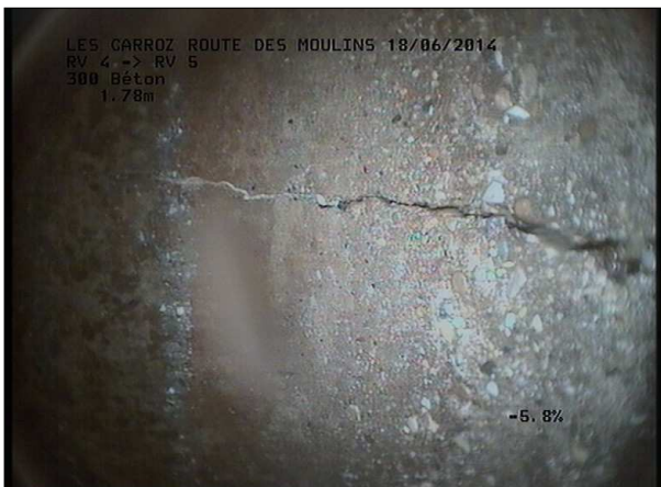
Photo: 4_2B, MPEG #: 180614_1, 00:00:16 1,78m, Fissure transversale (circulaire)
