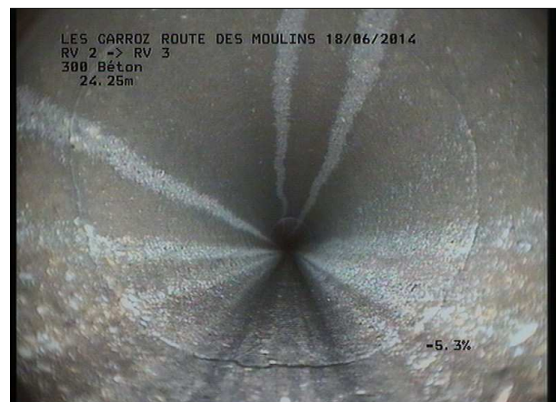
Photo: 2_7A, MPEG #: 180614_1, 00:03:01 24,51m, Fissure transversale (circulaire)
