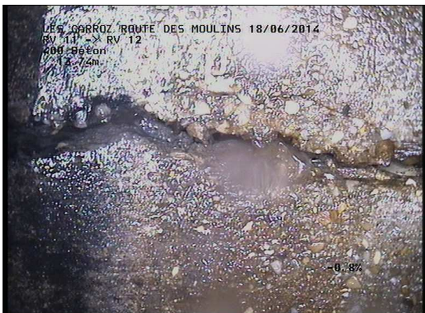
Photo: 11_4B, MPEG #: 180614_1, 00:01:55 13,74m, Fissure transversale (circulaire)
