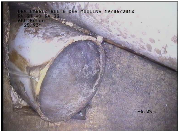
Photo: 21_5B, MPEG #: 180614_1, 00:02:26 25,93m, Raccordement direct à 09 h.
