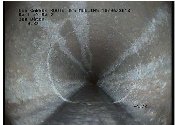
Photo: 1_2A, MPEG #: 180614_1, 00:00:30 4,22m, Fissure transversale (circulaire)
