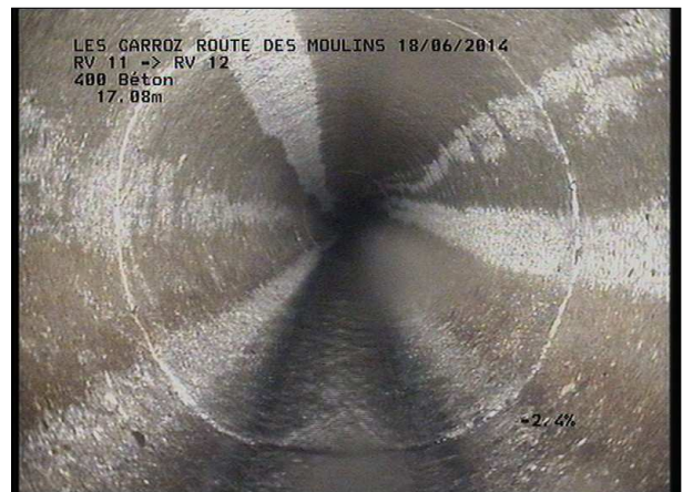
Photo: 11_5A, MPEG #: 180614_1, 00:02:29 17,55m, Fissure transversale (circulaire)
