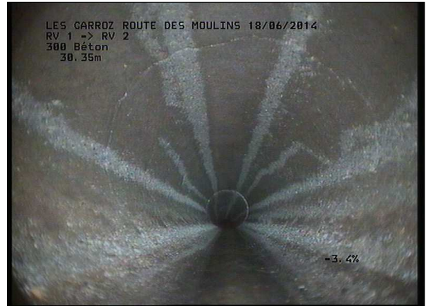
Photo: 1_13A, MPEG #: 180614_1, 00:05:13 30,57m, Fissure transversale (circulaire)
