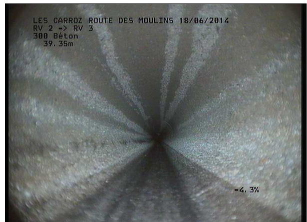
Photo: 2_9A, MPEG #: 180614_1, 00:04:34 39,64m, Fissure transversale (circulaire)
