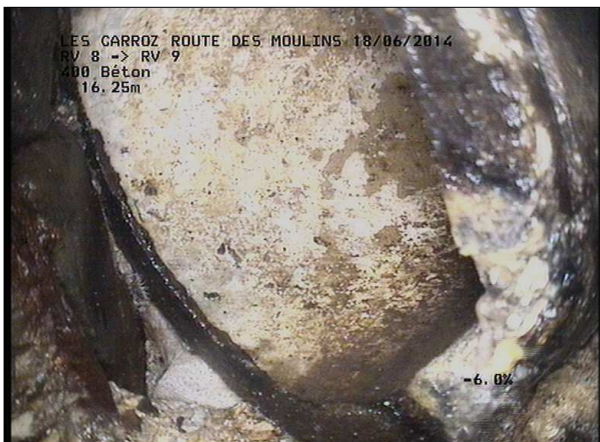
Photo: 8_6B, MPEG #: 180614_1, 00:02:52 16,25m, Raccordement direct à 01 h.
