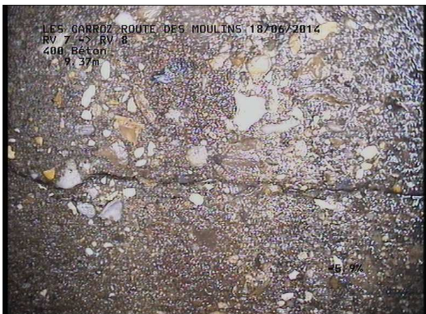
Photo: 7_4B, MPEG #: 180614_1, 00:01:30 9,37m, Fissure transversale (circulaire)
