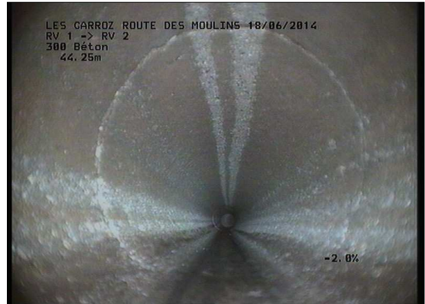
Photo: 1_17A, MPEG #: 180614_1, 00:07:19 44,47m, Fissure transversale (circulaire)
