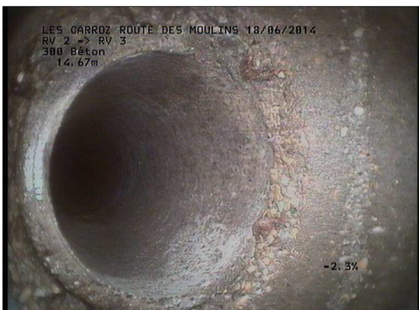
Photo: 2_6B, MPEG #: 180614_1, 00:02:14 14,67m, Raccordement direct à 10 h.
