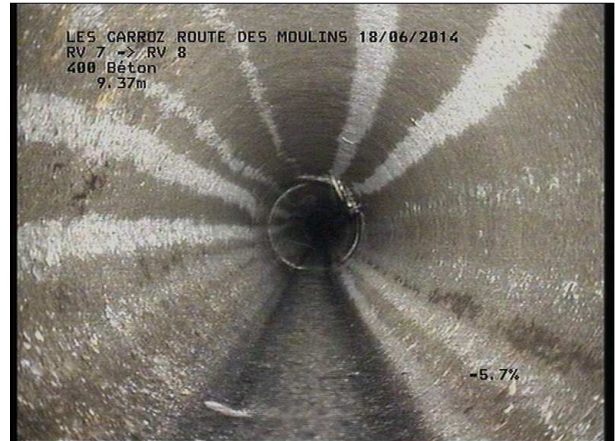
Photo: 7_4A, MPEG #: 180614_1, 00:01:30 9,37m, Fissure transversale (circulaire)
