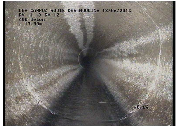
Photo: 11_4A, MPEG #: 180614_1, 00:01:55 13,74m, Fissure transversale (circulaire)
