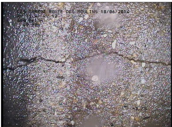
Photo: 11_8B, MPEG #: 180614_1, 00:04:36 29,9m, Fissure transversale (circulaire)
