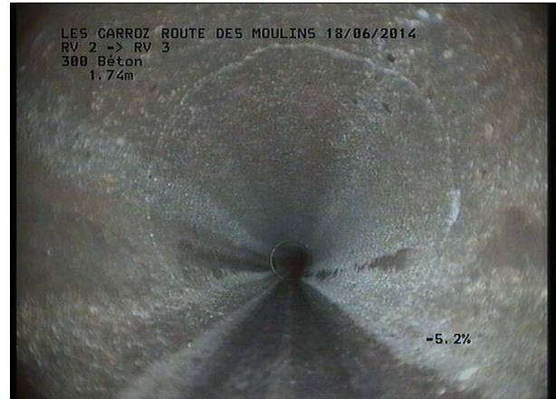
Photo: 2_2A, MPEG #: 180614_1, 00:00:14 2,03m, Fissure transversale (circulaire)
