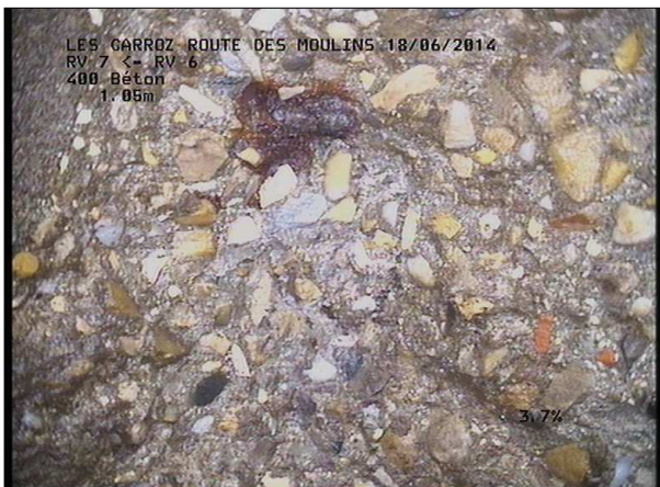
Photo: 6_2B, MPEG #: 180614_1, 00:00:05 1,05m, Perforation à 12 h.
