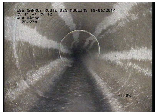
Photo: 11_7A, MPEG #: 180614_1, 00:03:56 26,41m, Fissure transversale (circulaire)
