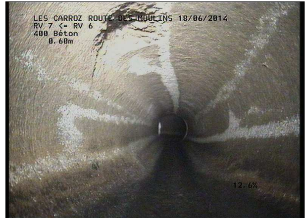
Photo: 6_2A, MPEG #: 180614_1, 00:00:05 1,05m, Perforation à 12 h.
