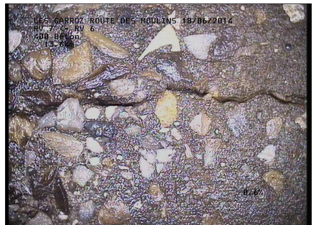
Photo: 6_5B, MPEG #: 180614_1, 00:02:44 13,64m, Fissure transversale (circulaire)
