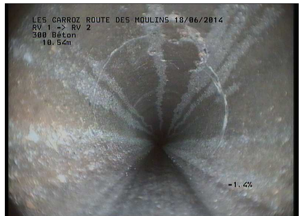
Photo: 1_8A, MPEG #: 180614_1, 00:02:34 10,86m, Fissure transversale (circulaire)
