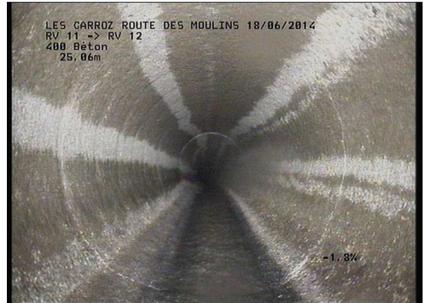
Photo: 11_6A, MPEG #: 180614_1, 00:03:32 25,5m, Fissure transversale (circulaire)
