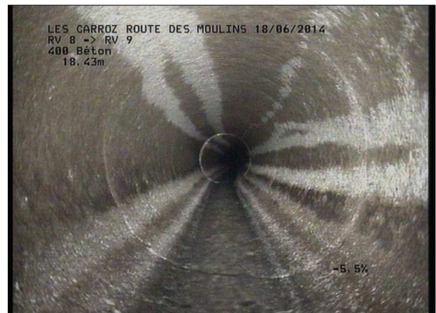
Photo: 8_7A, MPEG #: 180614_1, 00:03:22 18,97m, Fissure transversale (circulaire)
