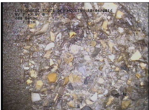
Photo: 7_2B, MPEG #: 180614_1, 00:00:39 7,81m, Perforation à 12 h.
