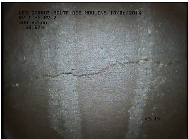
Photo: 1_13B, MPEG #: 180614_1, 00:05:13 30,57m, Fissure transversale (circulaire)
