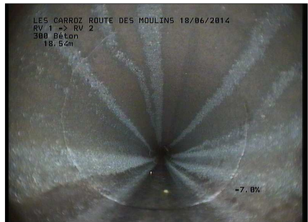
Photo: 1_10A, MPEG #: 180614_1, 00:03:44 18,82m, Fissure transversale (circulaire)
