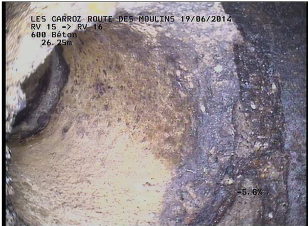
Photo: 15_3B, MPEG #: 180614_1, 00:02:05 26,25m, Raccordement direct à 11 h.
