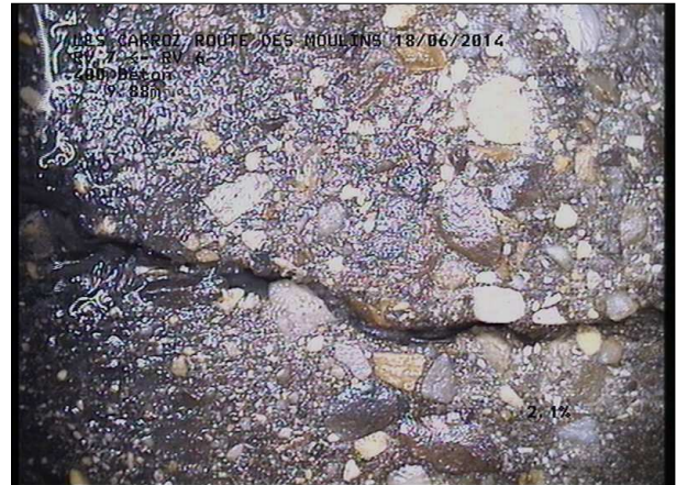
Photo: 6_4B, MPEG #: 180614_1, 00:01:36 9,88m, Fissure transversale (circulaire)
