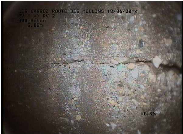
Photo: 1_3B, MPEG #: 180614_1, 00:00:52 5,05m, Fissure transversale (circulaire)
