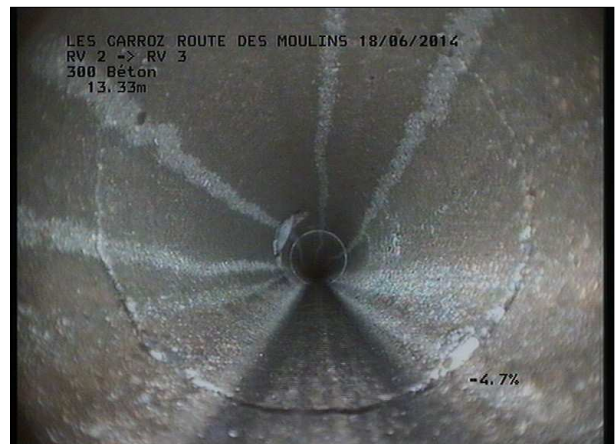
Photo: 2_5A, MPEG #: 180614_1, 00:01:47 13,57m, Fissure transversale (circulaire)
