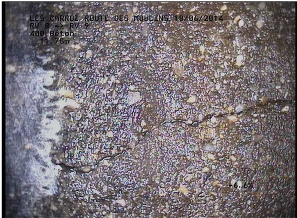
Photo: 8_3B, MPEG #: 180614_1, 00:01:20 11,75m, Fissure transversale (circulaire)
