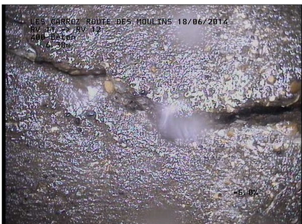
Photo: 11_2B, MPEG #: 180614_1, 00:00:40 6,38m, Fissure transversale (circulaire)
