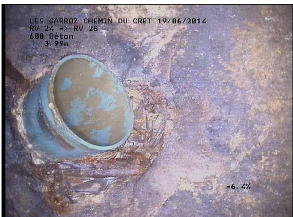
Photo: 24_2B, MPEG #: 180614_1, 00:00:13 3,99m, Raccordement direct à 11 h.
