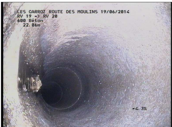
Photo: 19_3B, MPEG #: 180614_1, 00:01:23 22,06m, Raccordement direct à 09 h.
