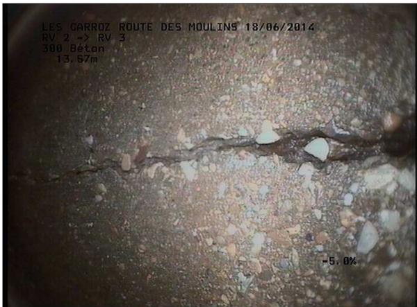
Photo: 2_5B, MPEG #: 180614_1, 00:01:47 13,57m, Fissure transversale (circulaire)
