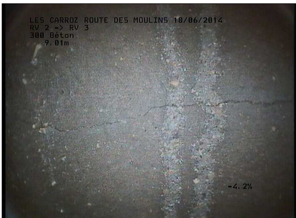
Photo: 2_4B, MPEG #: 180614_1, 00:01:13 9,01m, Fissure transversale (circulaire)
