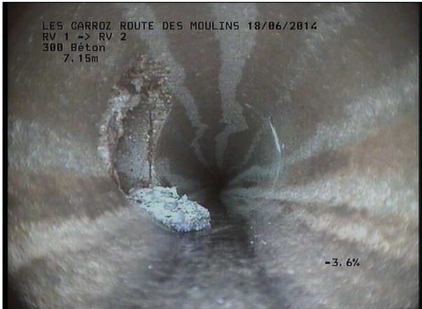
Photo: 1_6A, MPEG #: 180614_1, 00:01:51 7,6m, Raccordement direct à 09 h.
