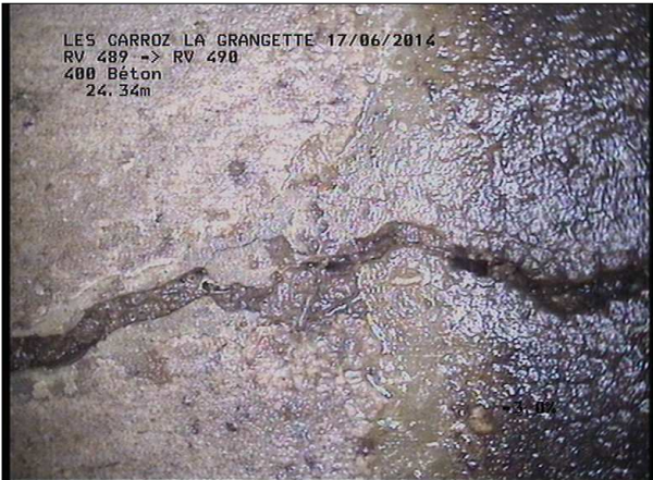
Photo: 11_7B, MPEG #: 160614_1, 00:06:29 23,72m, Fissure transversale (circulaire)
