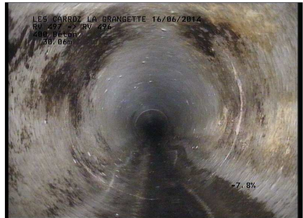
Photo: 4_12A, MPEG #: 160614_1, 00:07:23 30,69m, Fissure transversale (circulaire)
