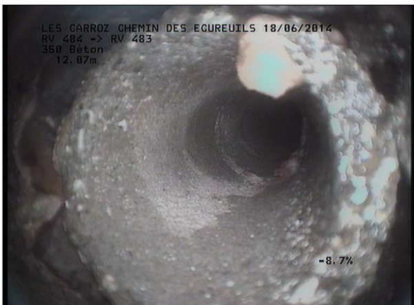
Photo: 23_2B, MPEG #: 160614_1, 00:01:07 12,07m, Raccordement direct à 03 h.
