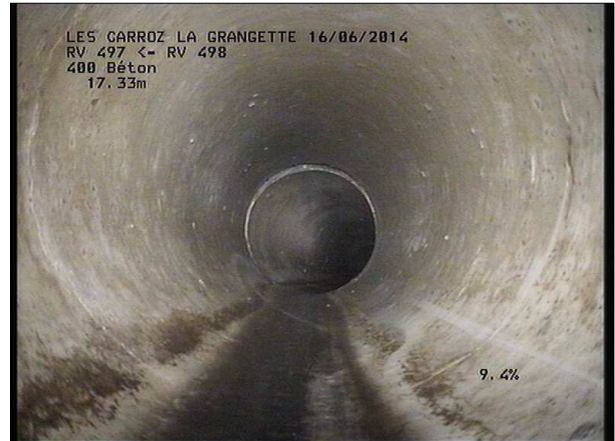
Photo: 1_9A, MPEG #: 160614_1, 00:04:21 17,64m, Fissure transversale (circulaire)
