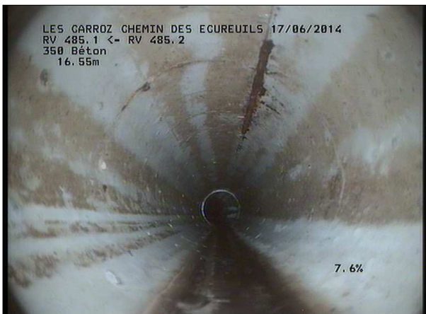
Photo: 18_6A, MPEG #: 160614_1, 00:02:42 16,87m, Fissure transversale (circulaire)
