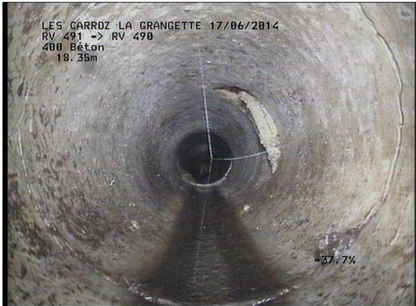
Photo: 10_12A, MPEG #: 160614_1, 00:05:30 18,69m, Fissure transversale (circulaire)
