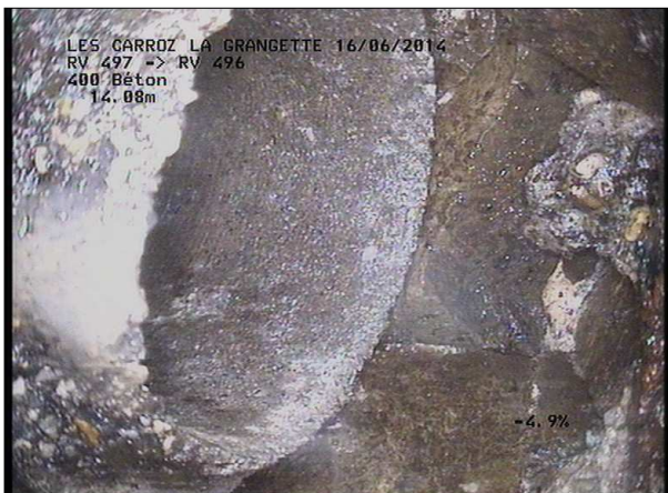
Photo: 4_4B, MPEG #: 160614_1, 00:01:57 14,08m, Raccordement direct à 11 h.
