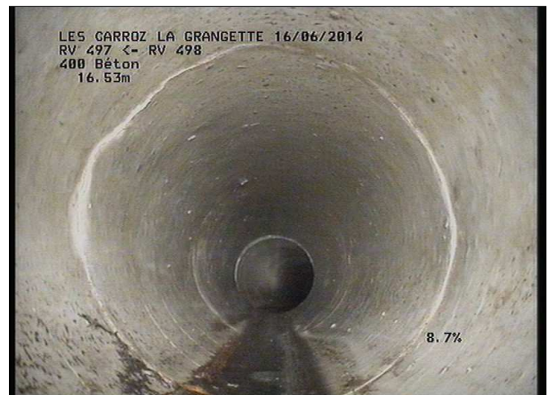
Photo: 1_8A, MPEG #: 160614_1, 00:03:49 17,11m, Fissure transversale (circulaire)
