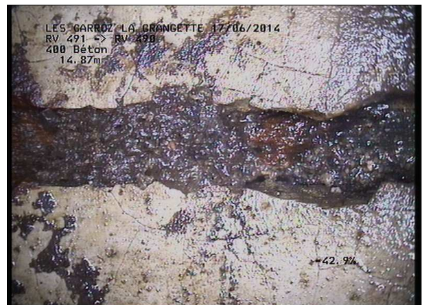
Photo: 10_11B, MPEG #: 160614_1, 00:04:54 14,87m, Fissure transversale (circulaire)
