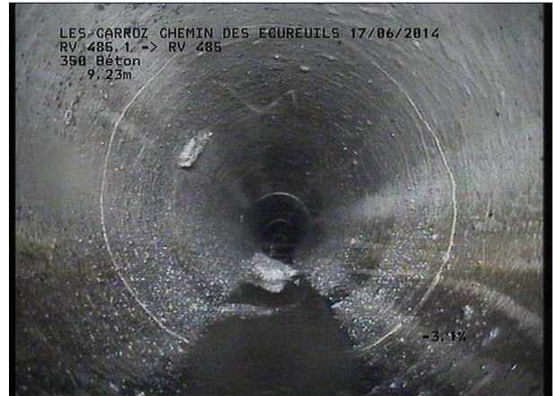
Photo: 19_4A, MPEG #: 160614_1, 00:01:40 9,81m, Fissure transversale (circulaire)
