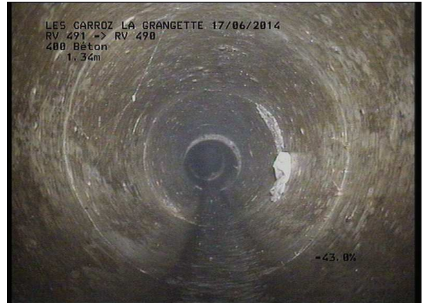
Photo: 10_2A, MPEG #: 160614_1, 00:00:19 1,79m, Fissure transversale (circulaire)
