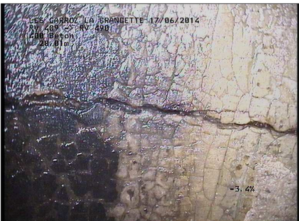
Photo: 11_8B, MPEG #: 160614_1, 00:07:35 27,38m, Fissure transversale (circulaire)
