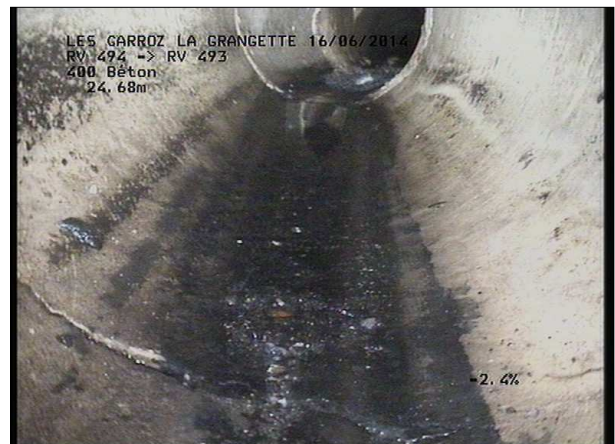
Photo: 7_9A, MPEG #: 160614_1, 00:05:45 24,68m, Fissure transversale (circulaire)
