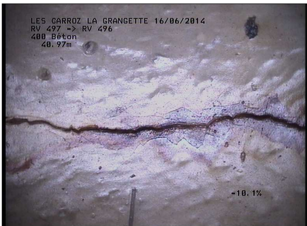
Photo: 4_16B, MPEG #: 160614_1, 00:09:47 40,97m, Fissure transversale (circulaire)
