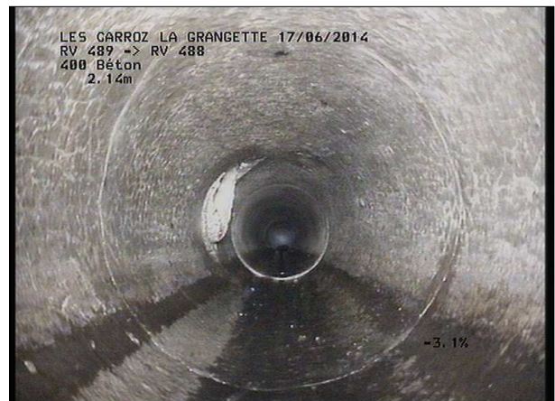
Photo: 12_3A, MPEG #: 160614_1, 00:00:37 2,14m, Fissure transversale (circulaire)
