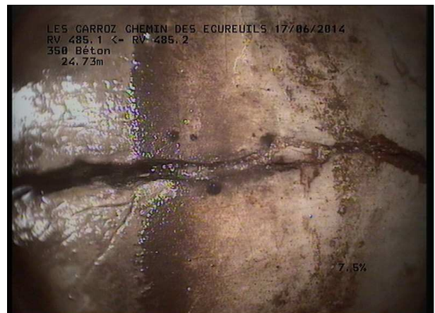
Photo: 18_8B, MPEG #: 160614_1, 00:04:08 24,73m, Fissure transversale (circulaire)
