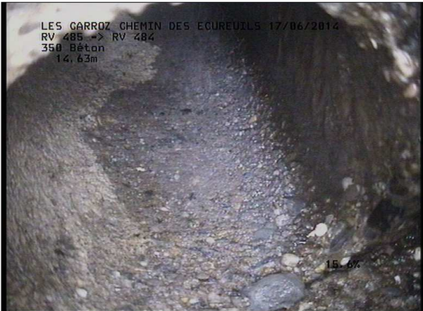
Photo: 20_5B, MPEG #: 160614_1, 00:01:45 14,1m, Raccordement direct à 03 h.
