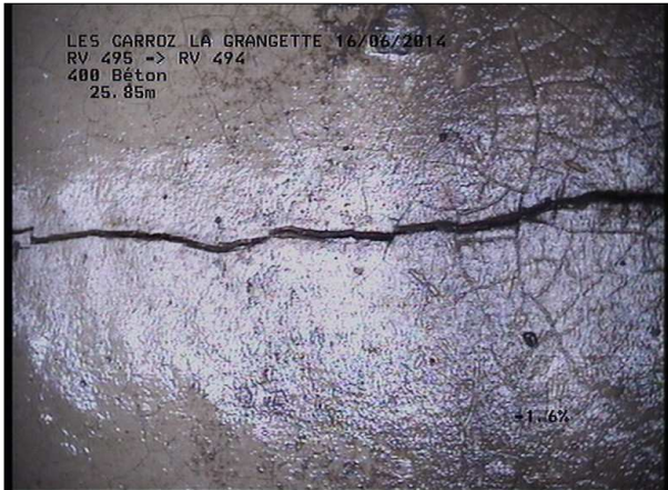
Photo: 6_5B, MPEG #: 160614_1, 00:03:16 25,85m, Fissure transversale (circulaire)
