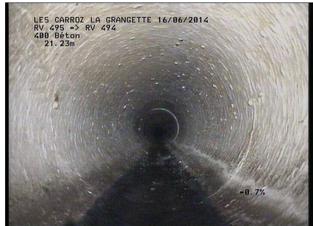
Photo: 6_4A, MPEG #: 160614_1, 00:02:31 21,86m, Fissure transversale (circulaire)
