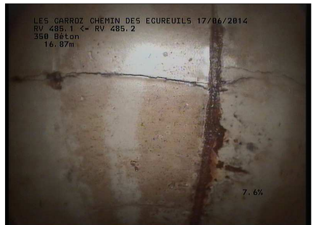
Photo: 18_6B, MPEG #: 160614_1, 00:02:42 16,87m, Fissure transversale (circulaire)
