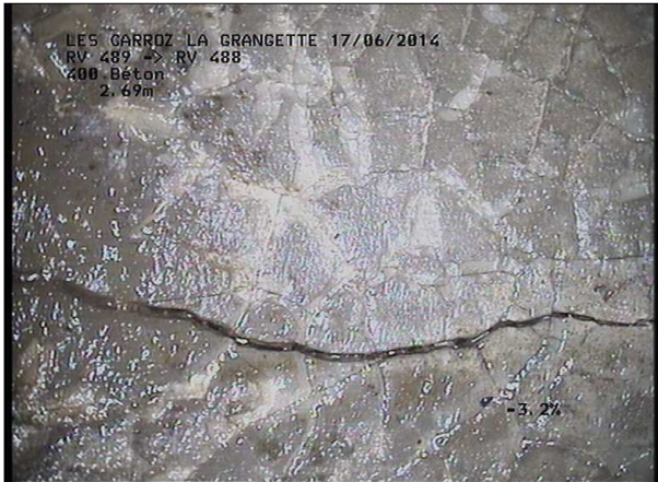
Photo: 12_3B, MPEG #: 160614_1, 00:00:37 2,14m, Fissure transversale (circulaire)
