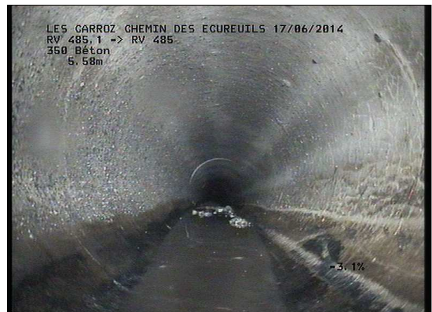
Photo: 19_3A, MPEG #: 160614_1, 00:00:52 6,06m, Fissure transversale (circulaire)
