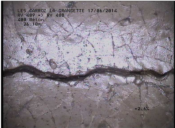
Photo: 12_9B, MPEG #: 160614_1, 00:05:41 26,1m, Fissure transversale (circulaire)
