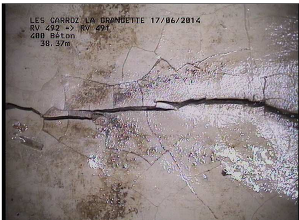
Photo: 9_17B, MPEG #: 160614_1, 00:07:49 38,36m, Fissure transversale (circulaire)
