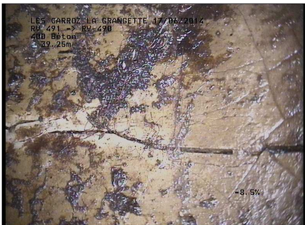
Photo: 10_21B, MPEG #: 160614_1, 00:09:31 39,25m, Fissure transversale (circulaire)
