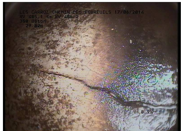
Photo: 18_10B, MPEG #: 160614_1, 00:05:17 29,82m, Fissure transversale (circulaire)
