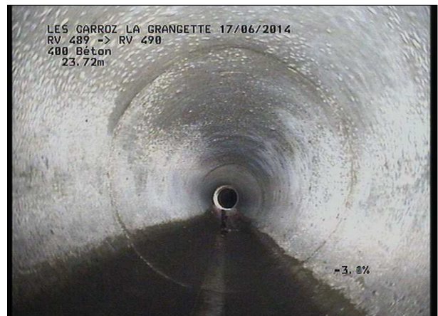
Photo: 11_7A, MPEG #: 160614_1, 00:06:29 23,72m, Fissure transversale (circulaire)
