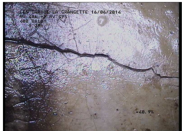
Photo: 5_5B, MPEG #: 160614_1, 00:01:46 9,29m, Fissure transversale (circulaire)
