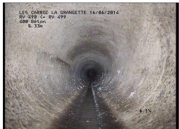
Photo: 2_3A, MPEG #: 160614_1, 00:01:09 5,91m, Fissure transversale (circulaire)
