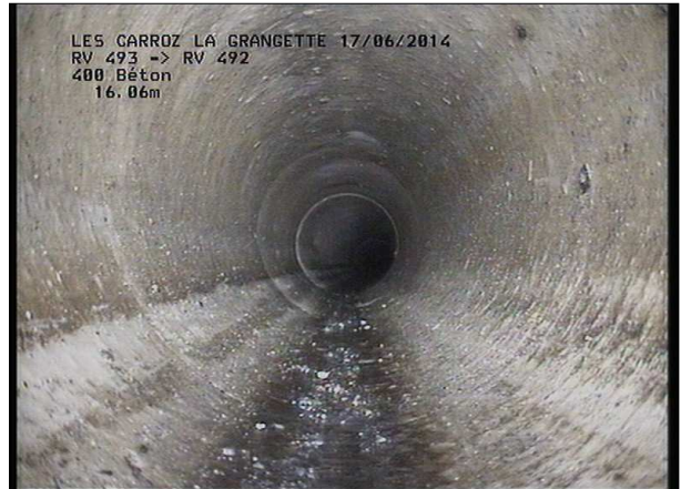
Photo: 8_6A, MPEG #: 160614_1, 00:02:39 16,61m, Fissure transversale (circulaire)
