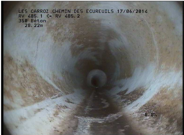
Photo: 18_9A, MPEG #: 160614_1, 00:04:48 28,49m, Fissure transversale (circulaire)
