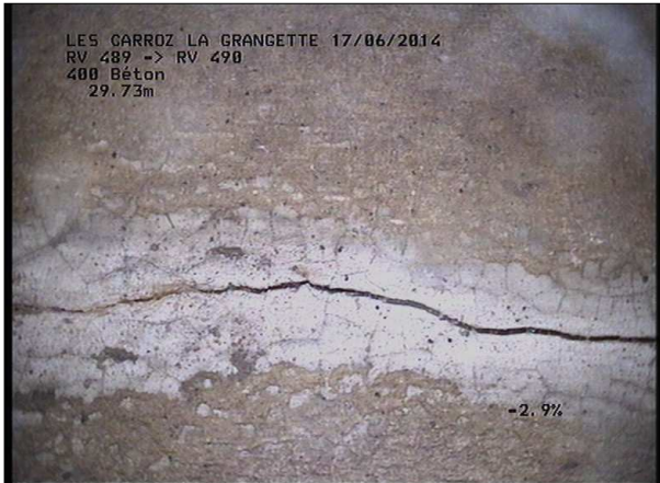
Photo: 11_9B, MPEG #: 160614_1, 00:08:12 29,73m, Fissure transversale (circulaire)
