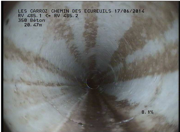
Photo: 18_7A, MPEG #: 160614_1, 00:03:25 20,71m, Fissure transversale (circulaire)
