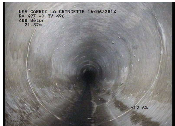
Photo: 4_7A, MPEG #: 160614_1, 00:03:59 22,28m, Fissure transversale (circulaire)
