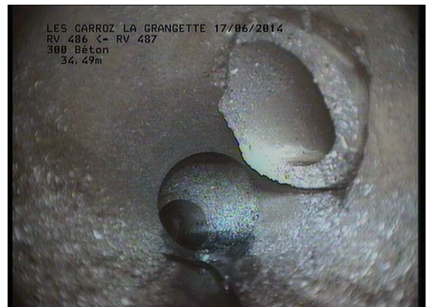
Photo: 15_9A, MPEG #: 160614_1, 00:00:36 34,74m, Raccordement direct à 01 h.
