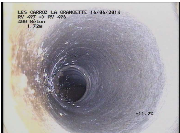
Photo: 4_2B, MPEG #: 160614_1, 00:00:11 1,72m, Raccordement direct à 11 h.
