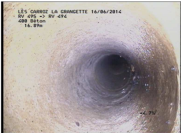
Photo: 6_3B, MPEG #: 160614_1, 00:01:46 16,89m, Raccordement direct à 02 h.
