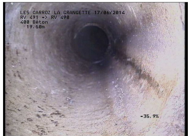
Photo: 10_13B, MPEG #: 160614_1, 00:05:53 19,5m, Raccordement direct à 02 h.
