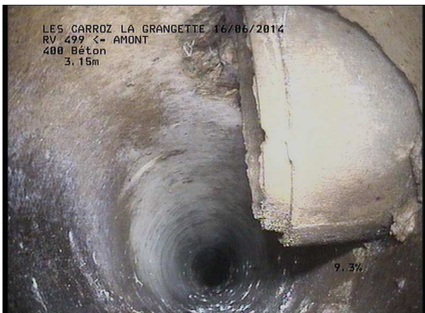
Photo: 3_3A, MPEG #: 160614_1, 00:05:20 3,15m, Interruption de l'inspection franchissement raccordement pénétrant impossible
