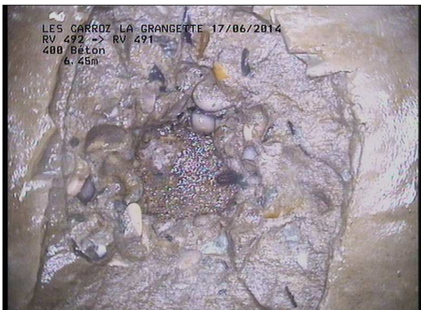
Photo: 9_2B, MPEG #: 160614_1, 00:00:33 6,45m, Perforation à 11 h.
