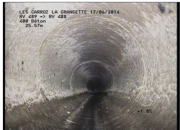
Photo: 12_9A, MPEG #: 160614_1, 00:05:41 26,1m, Fissure transversale (circulaire)
