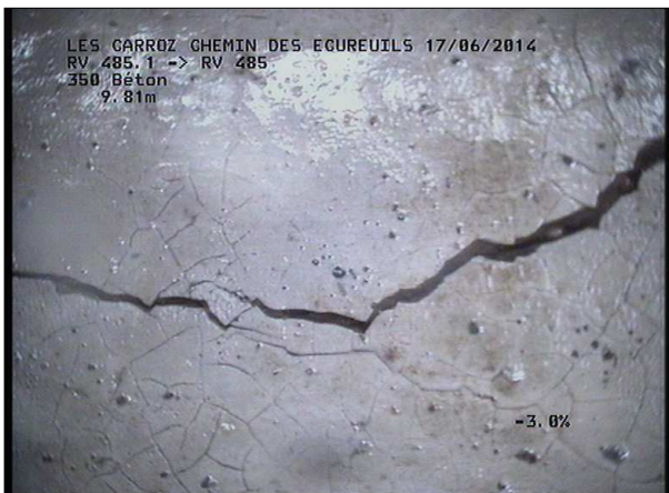
Photo: 19_4B, MPEG #: 160614_1, 00:01:40 9,81m, Fissure transversale (circulaire)
