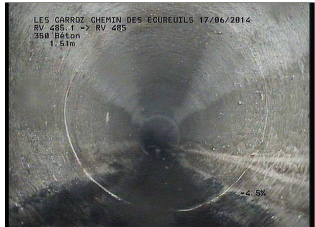
Photo: 19_2A, MPEG #: 160614_1, 00:00:16 2,07m, Fissure transversale (circulaire)
