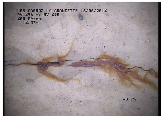
Photo: 5_7B, MPEG #: 160614_1, 00:02:48 14,33m, Fissure transversale (circulaire)
