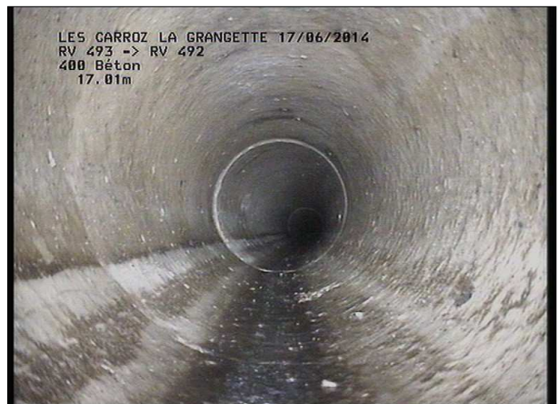
Photo: 8_7A, MPEG #: 160614_1, 00:03:03 17,47m, Fissure transversale (circulaire)
