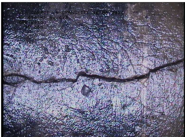
Photo: 7_4B, MPEG #: 160614_1, 00:02:33 15,66m, Fissure transversale (circulaire)
