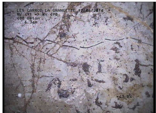
Photo: 10_7B, MPEG #: 160614_1, 00:02:27 6,34m, Fissure transversale (circulaire)
