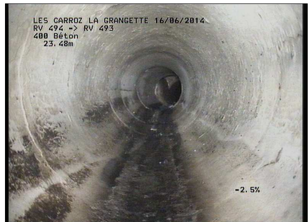
Photo: 7_7A, MPEG #: 160614_1, 00:05:00 23,83m, Fissure transversale (circulaire)
