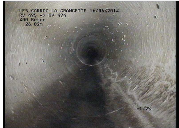
Photo: 6_6A, MPEG #: 160614_1, 00:03:41 26,54m, Fissure transversale (circulaire)
