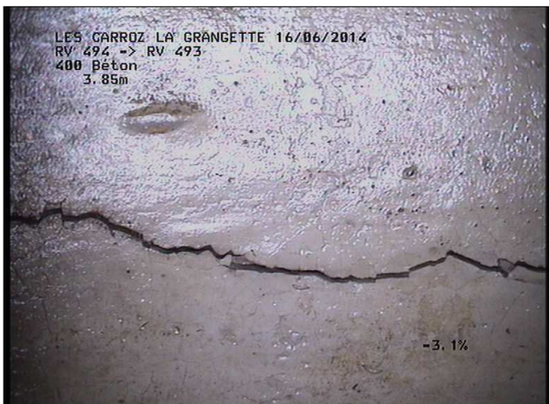
Photo: 7_2B, MPEG #: 160614_1, 00:00:26 3,85m, Fissure transversale (circulaire)
