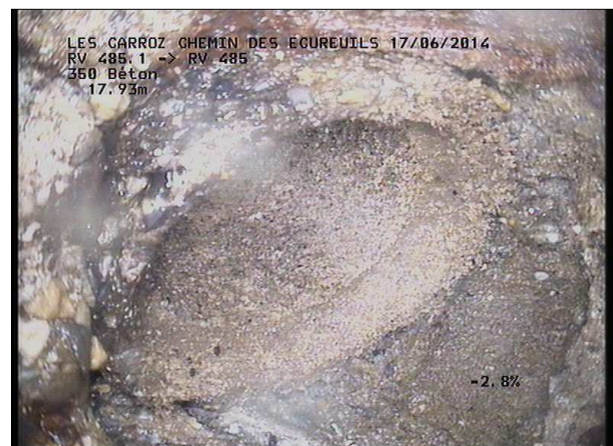
Photo: 19_7B, MPEG #: 160614_1, 00:03:51 17,93m, Raccordement direct à 11 h.
