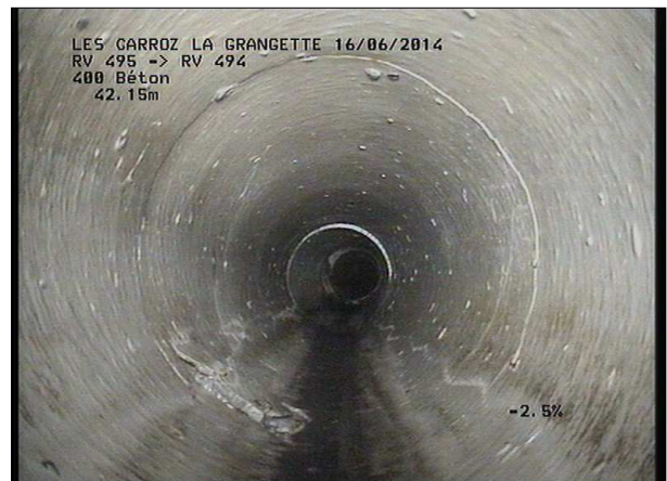
Photo: 6_11A, MPEG #: 160614_1, 00:07:04 42,63m, Fissure transversale (circulaire)
