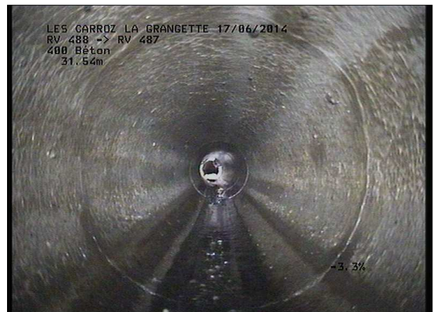
Photo: 13_10A, MPEG #: 160614_1, 00:05:31 32,03m, Fissure transversale (circulaire)
