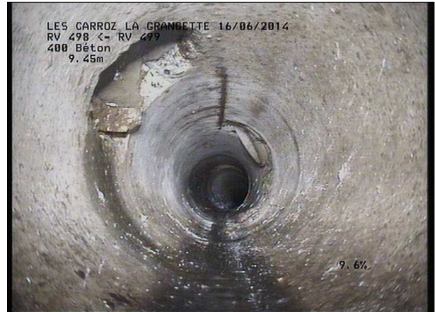
Photo: 2_5A, MPEG #: 160614_1, 00:02:16 10,1m, Raccordement direct à 10 h.
