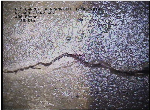
Photo: 13_8B, MPEG #: 160614_1, 00:04:05 23,89m, Fissure transversale (circulaire)
