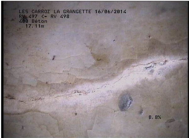
Photo: 1_8B, MPEG #: 160614_1, 00:03:49 17,11m, Fissure transversale (circulaire)
