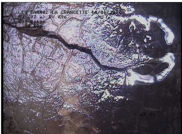
Photo: 4_12B, MPEG #: 160614_1, 00:07:23 30,69m, Fissure transversale (circulaire)
