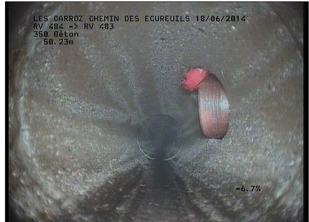
Photo: 23_12A, MPEG #: 160614_1, 00:08:18 50,78m, Raccordement direct à 01 h.
