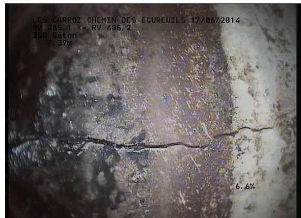
Photo: 18_4B, MPEG #: 160614_1, 00:01:40 7,39m, Fissure transversale (circulaire)
