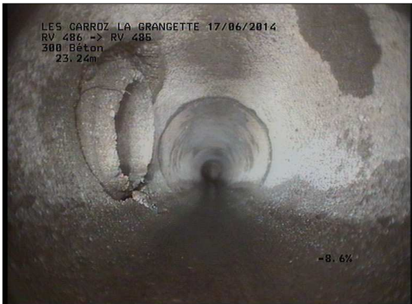
Photo: 16_6A, MPEG #: 160614_1, 00:02:47 23,59m, Raccordement direct à 09 h.
