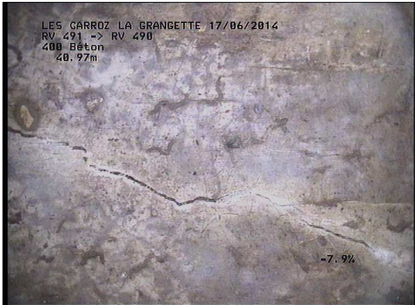
Photo: 10_22B, MPEG #: 160614_1, 00:09:59 40,47m, Fissure transversale (circulaire)
