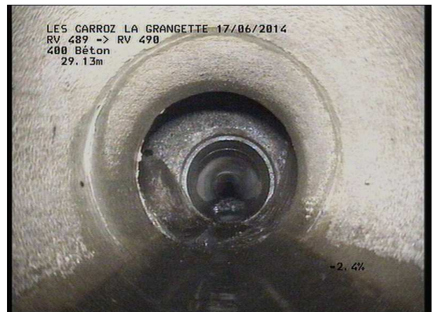
Photo: 11_9A, MPEG #: 160614_1, 00:08:12 29,73m, Fissure transversale (circulaire)
