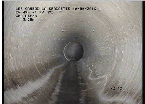
Photo: 7_2A, MPEG #: 160614_1, 00:00:26 3,85m, Fissure transversale (circulaire)
