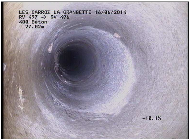
Photo: 4_11B, MPEG #: 160614_1, 00:06:21 27,02m, Raccordement direct à 11 h.
