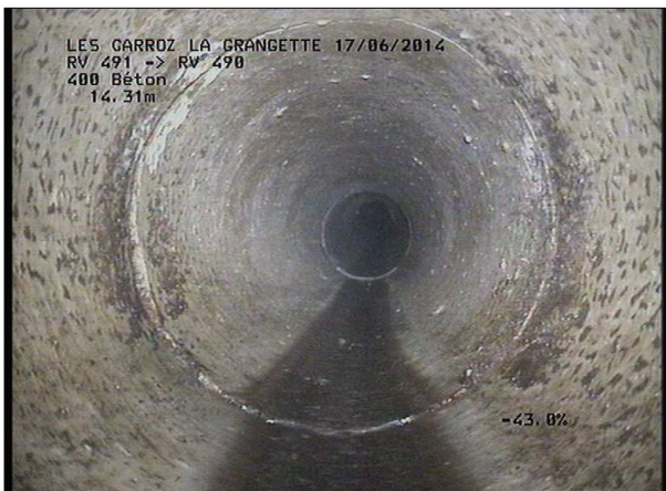
Photo: 10_11A, MPEG #: 160614_1, 00:04:54 14,87m, Fissure transversale (circulaire)
