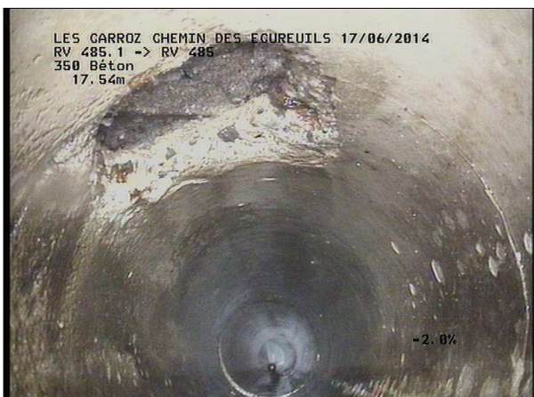
Photo: 19_7A, MPEG #: 160614_1, 00:03:51 17,93m, Raccordement direct à 11 h.
