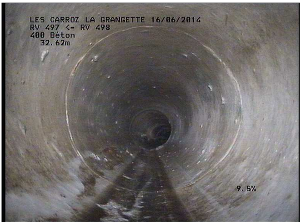
Photo: 1_13A, MPEG #: 160614_1, 00:07:17 33,26m, Fissure transversale (circulaire)
