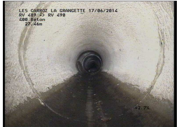
Photo: 11_8A, MPEG #: 160614_1, 00:07:35 27,38m, Fissure transversale (circulaire)
