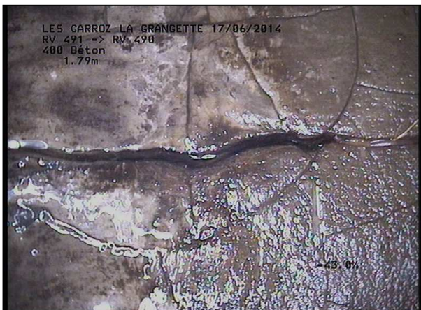
Photo: 10_2B, MPEG #: 160614_1, 00:00:19 1,79m, Fissure transversale (circulaire)
