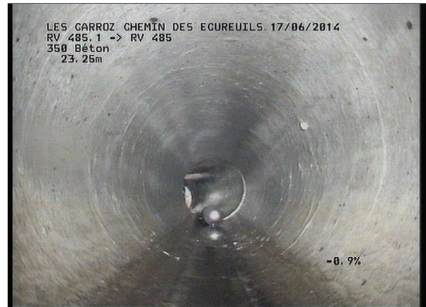
Photo: 19_9A, MPEG #: 160614_1, 00:04:53 23,77m, Fissure transversale (circulaire)
