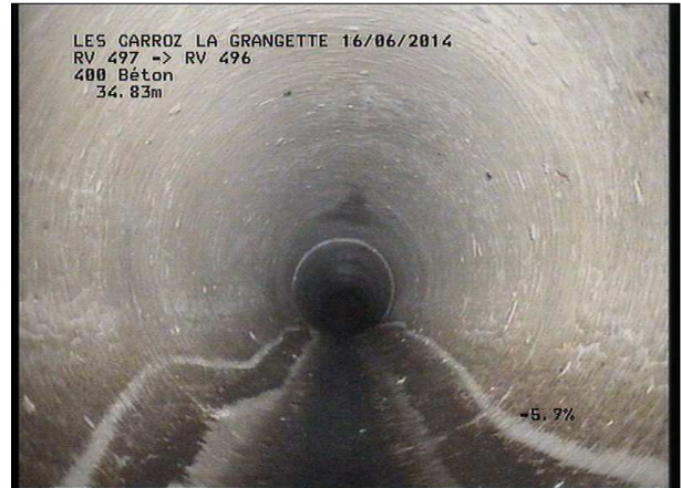
Photo: 4_14A, MPEG #: 160614_1, 00:08:38 35,44m, Fissure transversale (circulaire)
