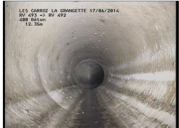
Photo: 8_4A, MPEG #: 160614_1, 00:01:37 12,95m, Fissure transversale (circulaire)
