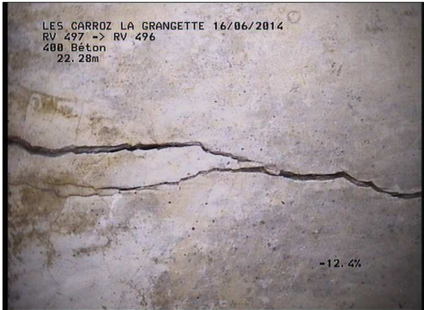
Photo: 4_7B, MPEG #: 160614_1, 00:03:59 22,28m, Fissure transversale (circulaire)
