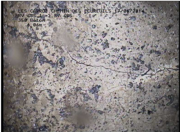
Photo: 19_3B, MPEG #: 160614_1, 00:00:52 6,06m, Fissure transversale (circulaire)
