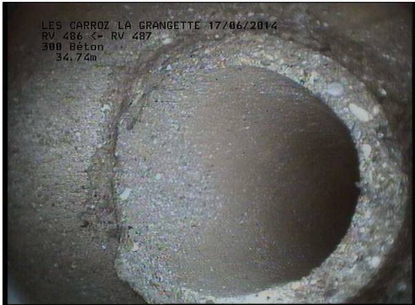
Photo: 15_9B, MPEG #: 160614_1, 00:00:36 34,74m, Raccordement direct à 01 h.
