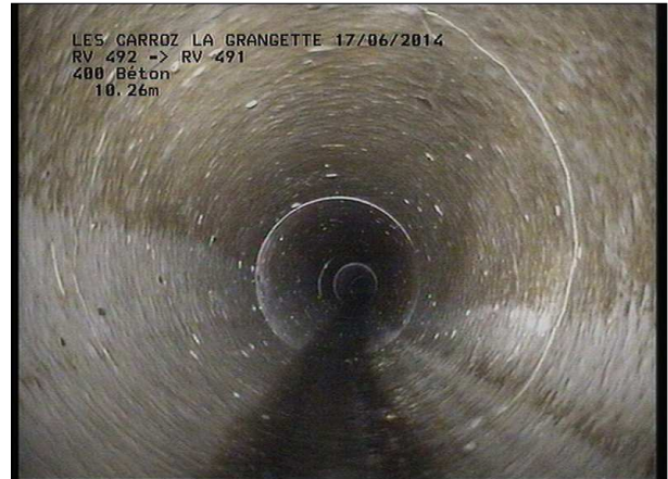
Photo: 9_4A, MPEG #: 160614_1, 00:01:21 10,74m, Fissure transversale (circulaire)
