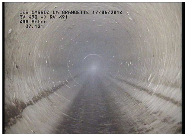
Photo: 9_16A, MPEG #: 160614_1, 00:07:27 37,57m, Fissure transversale (circulaire)
