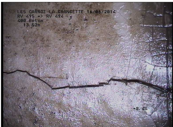
Photo: 6_2B, MPEG #: 160614_1, 00:01:11 13,52m, Fissure transversale (circulaire)
