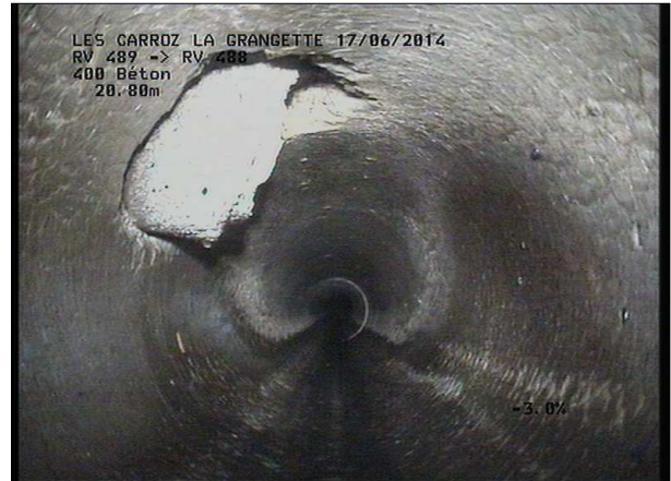
Photo: 12_8A, MPEG #: 160614_1, 00:04:31 21,49m, Raccordement direct à 11 h.
