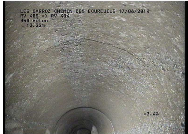
Photo: 20_4A, MPEG #: 160614_1, 00:01:45 12,67m, Fissure transversale (circulaire)
