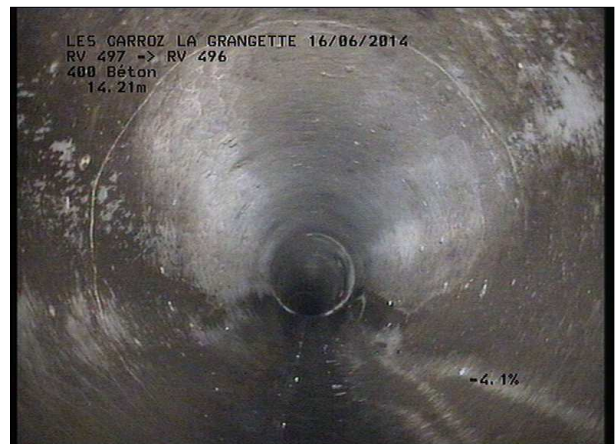
Photo: 4_5A, MPEG #: 160614_1, 00:02:22 14,75m, Fissure transversale (circulaire)
