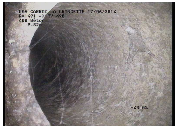
Photo: 10_9B, MPEG #: 160614_1, 00:03:51 9,82m, Raccordement direct à 11 h.
