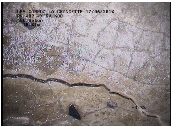
Photo: 12_6B, MPEG #: 160614_1, 00:02:32 10,41m, Fissure transversale (circulaire)
