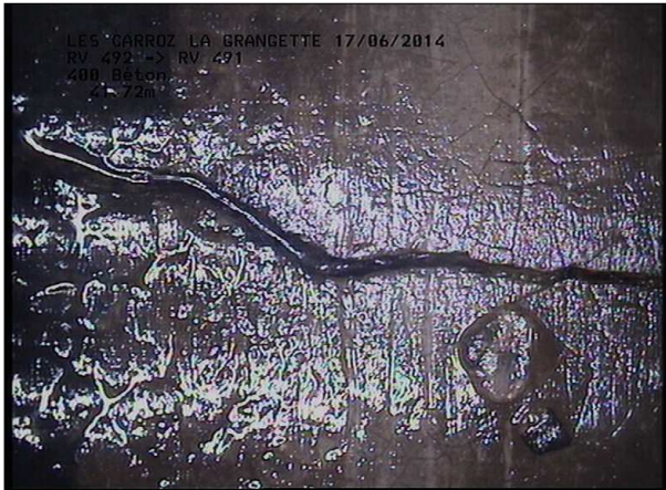
Photo: 9_18B, MPEG #: 160614_1, 00:08:42 41,72m, Fissure transversale (circulaire)
