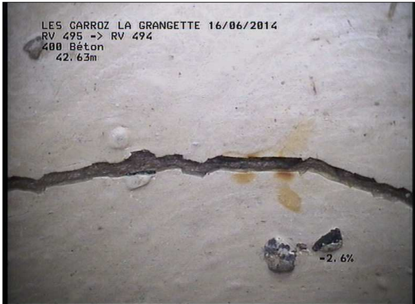
Photo: 6_11B, MPEG #: 160614_1, 00:07:04 42,63m, Fissure transversale (circulaire)
