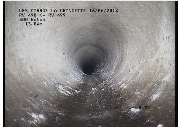
Photo: 2_10A, MPEG #: 160614_1, 00:04:40 14,31m, Fissure transversale (circulaire)
