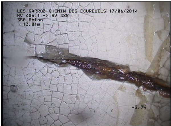
Photo: 19_5B, MPEG #: 160614_1, 00:03:11 13,81m, Fissure transversale (circulaire)
