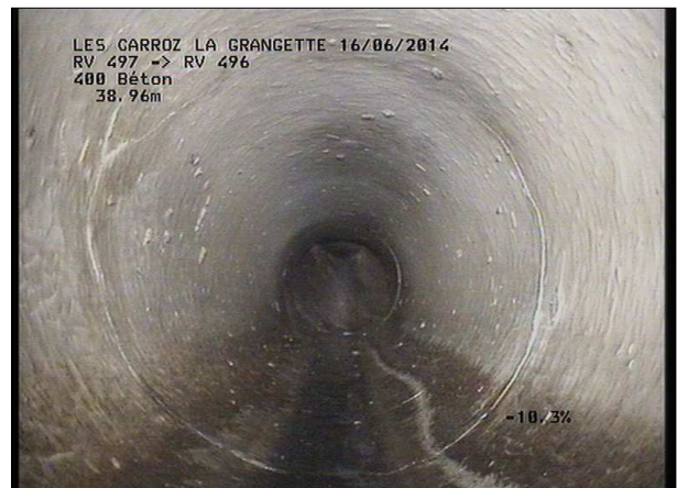
Photo: 4_15A, MPEG #: 160614_1, 00:09:17 39,51m, Fissure transversale (circulaire)
