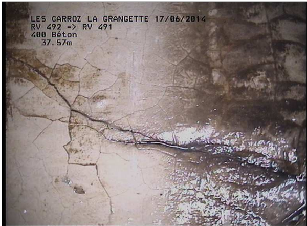
Photo: 9_16B, MPEG #: 160614_1, 00:07:27 37,57m, Fissure transversale (circulaire)
