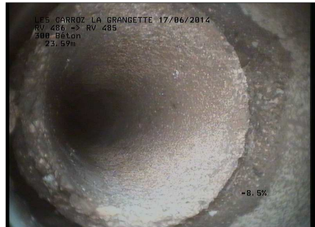
Photo: 16_6B, MPEG #: 160614_1, 00:02:47 23,59m, Raccordement direct à 09 h.
