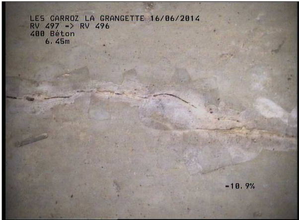
Photo: 4_3B, MPEG #: 160614_1, 00:00:54 5,95m, Fissure transversale (circulaire)
