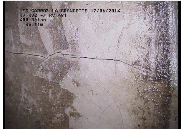
Photo: 9_21B, MPEG #: 160614_1, 00:10:07 45,11m, Fissure transversale (circulaire)
