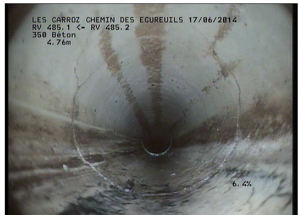
Photo: 18_3A, MPEG #: 160614_1, 00:01:09 5,08m, Fissure transversale (circulaire)
