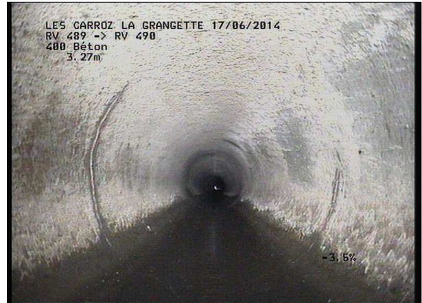
Photo: 11_2A, MPEG #: 160614_1, 00:00:21 3,27m, Fissure transversale (circulaire)
