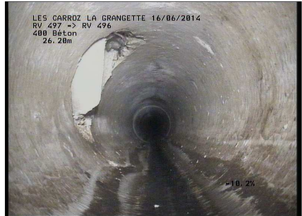
Photo: 4_10A, MPEG #: 160614_1, 00:05:51 26,74m, Fissure transversale (circulaire)
