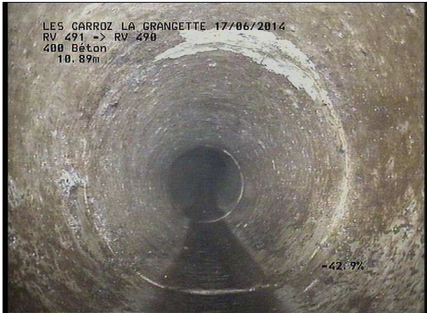
Photo: 10_10A, MPEG #: 160614_1, 00:04:18 11,48m, Fissure transversale (circulaire)
