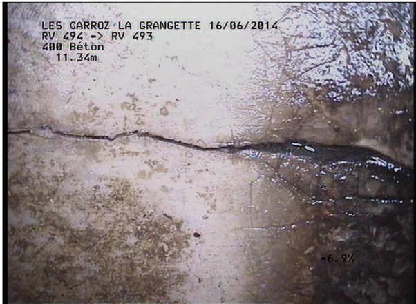
Photo: 7_3B, MPEG #: 160614_1, 00:01:35 11,34m, Fissure transversale (circulaire)
