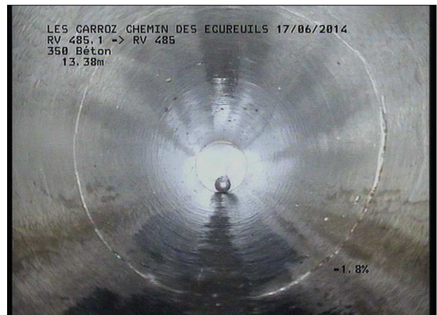
Photo: 19_5A, MPEG #: 160614_1, 00:03:11 13,81m, Fissure transversale (circulaire)
