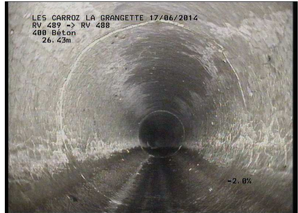
Photo: 12_10A, MPEG #: 160614_1, 00:06:15 26,95m, Fissure transversale (circulaire)
