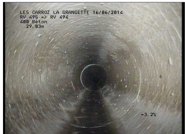
Photo: 6_7A, MPEG #: 160614_1, 00:04:20 30,45m, Fissure transversale (circulaire)
