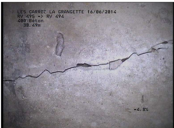
Photo: 6_10B, MPEG #: 160614_1, 00:06:02 38,49m, Fissure transversale (circulaire)
