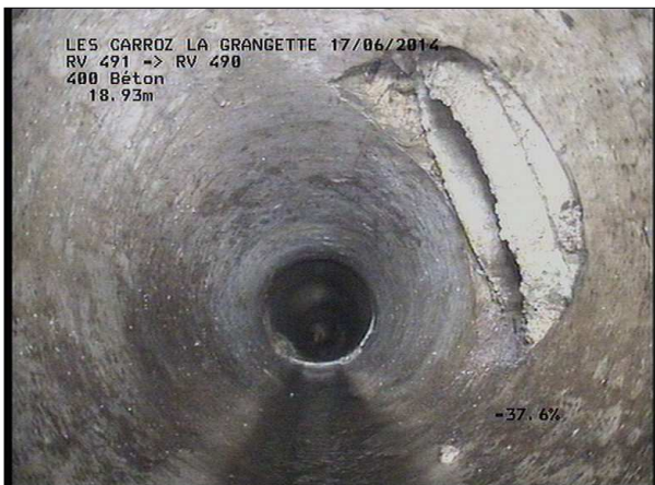
Photo: 10_13A, MPEG #: 160614_1, 00:05:53 19,5m, Raccordement direct à 02 h.
