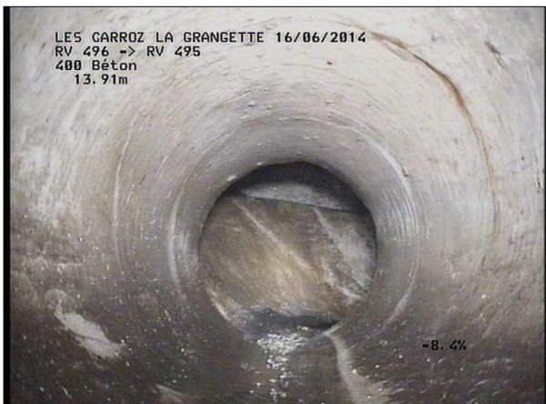
Photo: 5_7A, MPEG #: 160614_1, 00:02:48 14,33m, Fissure transversale (circulaire)
