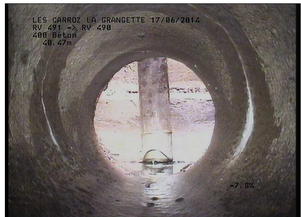
Photo: 10_22A, MPEG #: 160614_1, 00:09:59 40,47m, Fissure transversale (circulaire)
