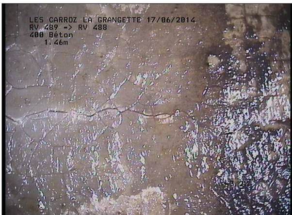
Photo: 12_2B, MPEG #: 160614_1, 00:00:11 1,46m, Fissure transversale (circulaire)
