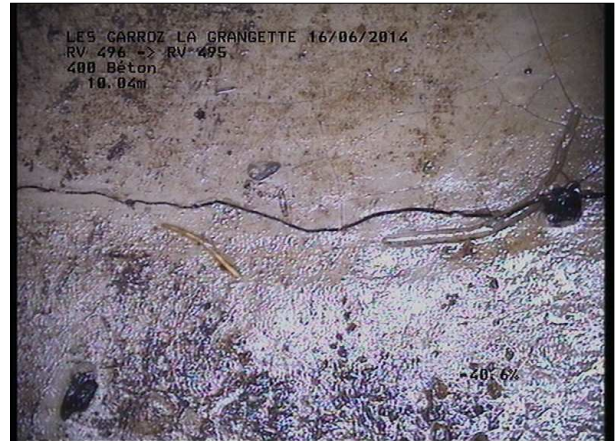
Photo: 5_6B, MPEG #: 160614_1, 00:02:08 10,04m, Fissure transversale (circulaire)
