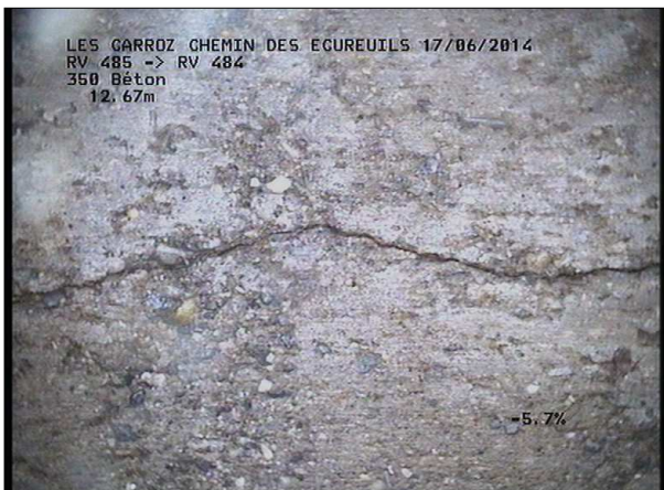
Photo: 20_4B, MPEG #: 160614_1, 00:01:45 12,67m, Fissure transversale (circulaire)
