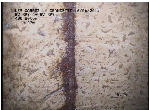
Photo: 2_2B, MPEG #: 160614_1, 00:00:40 4,49m, Armatures visibles à 10 h.
