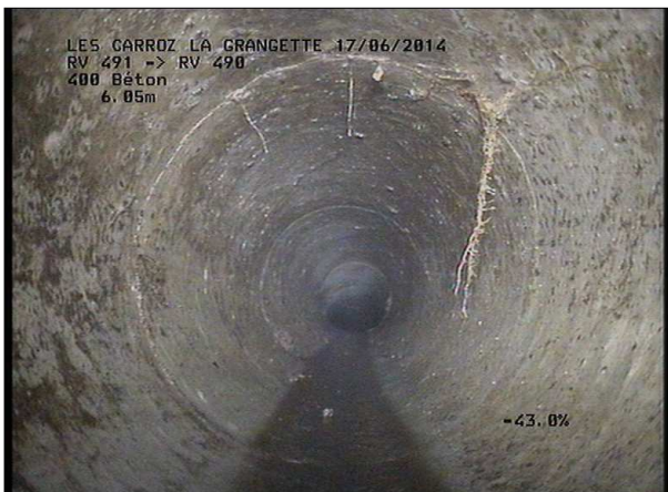
Photo: 10_7A, MPEG #: 160614_1, 00:02:27 6,34m, Fissure transversale (circulaire)
