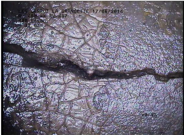
Photo: 13_10B, MPEG #: 160614_1, 00:05:31 32,03m, Fissure transversale (circulaire)
