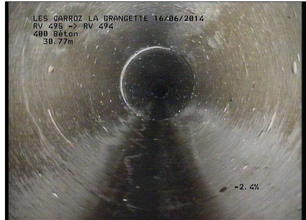
Photo: 6_8A, MPEG #: 160614_1, 00:04:44 31,18m, Fissure transversale (circulaire)
