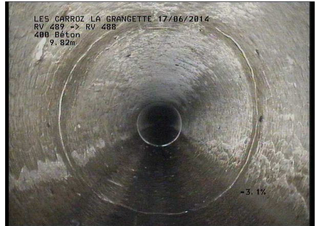
Photo: 12_6A, MPEG #: 160614_1, 00:02:32 10,41m, Fissure transversale (circulaire)
