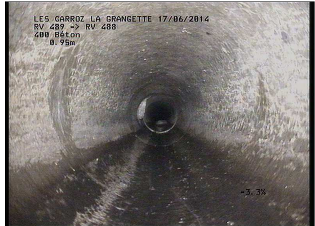
Photo: 12_2A, MPEG #: 160614_1, 00:00:11 1,46m, Fissure transversale (circulaire)
