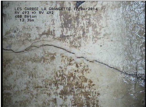
Photo: 8_3B, MPEG #: 160614_1, 00:01:20 12,35m, Fissure transversale (circulaire)
