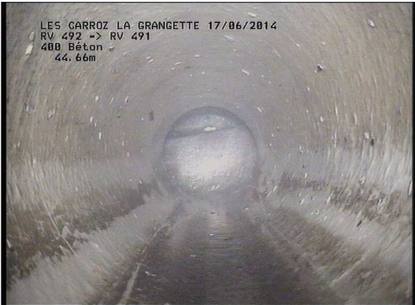
Photo: 9_21A, MPEG #: 160614_1, 00:10:07 45,11m, Fissure transversale (circulaire)
