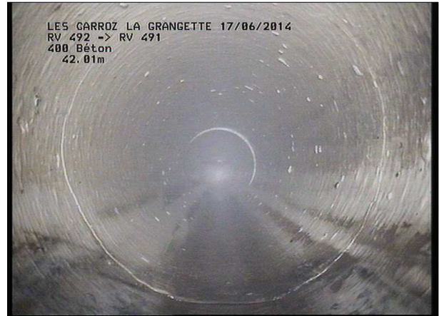
Photo: 9_19A, MPEG #: 160614_1, 00:09:12 42,51m, Fissure transversale (circulaire)
