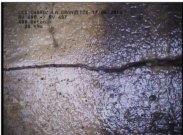
Photo: 13_9B, MPEG #: 160614_1, 00:04:53 28,19m, Fissure transversale (circulaire)
