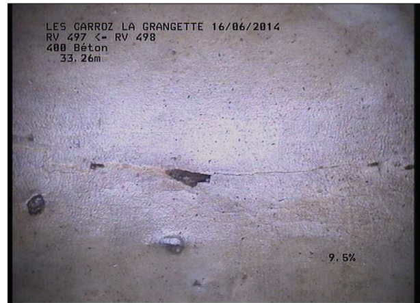
Photo: 1_13B, MPEG #: 160614_1, 00:07:17 33,26m, Fissure transversale (circulaire)
