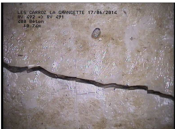
Photo: 9_4B, MPEG #: 160614_1, 00:01:21 10,74m, Fissure transversale (circulaire)
