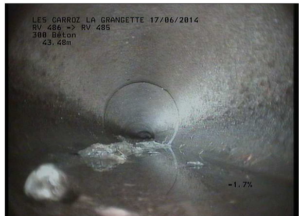
Photo: 16_15A, MPEG #: 160614_1, 00:07:51 43,48m, Interruption de l'inspection
