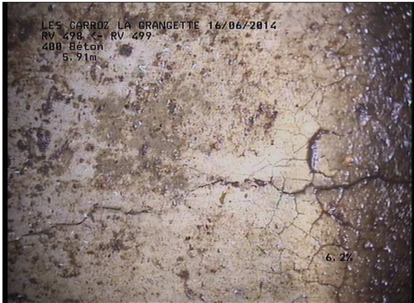
Photo: 2_3B, MPEG #: 160614_1, 00:01:09 5,91m, Fissure transversale (circulaire)
