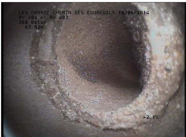
Photo: 23_14B, MPEG #: 160614_1, 00:09:58 63,02m, Raccordement direct à 03 h.
