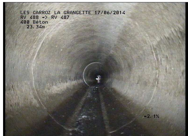
Photo: 13_8A, MPEG #: 160614_1, 00:04:05 23,89m, Fissure transversale (circulaire)
