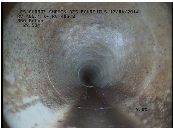
Photo: 18_10A, MPEG #: 160614_1, 00:05:17 29,82m, Fissure transversale (circulaire)
