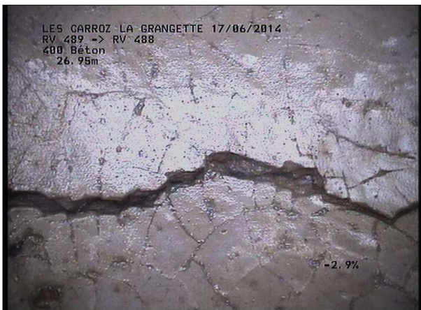
Photo: 12_10B, MPEG #: 160614_1, 00:06:15 26,95m, Fissure transversale (circulaire)
