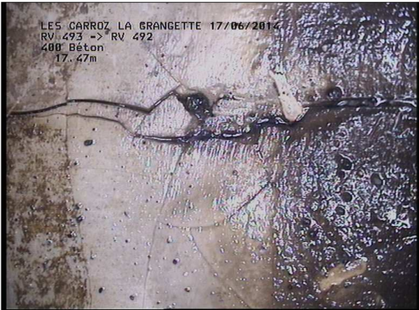
Photo: 8_7B, MPEG #: 160614_1, 00:03:03 17,47m, Fissure transversale (circulaire)
