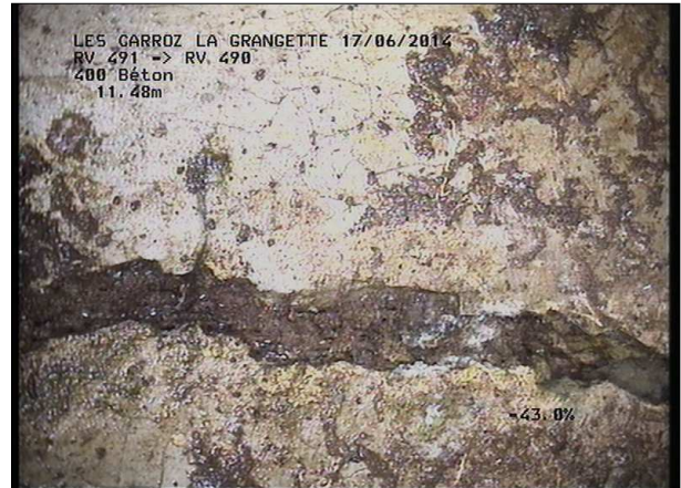
Photo: 10_10B, MPEG #: 160614_1, 00:04:18 11,48m, Fissure transversale (circulaire)
