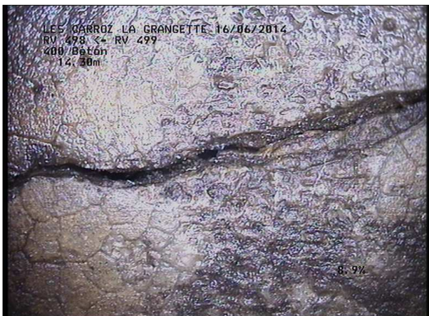
Photo: 2_10B, MPEG #: 160614_1, 00:04:40 14,31m, Fissure transversale (circulaire)
