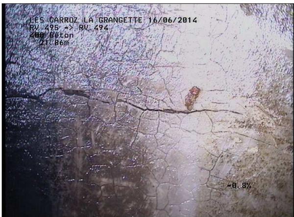
Photo: 6_4B, MPEG #: 160614_1, 00:02:31 21,86m, Fissure transversale (circulaire)
