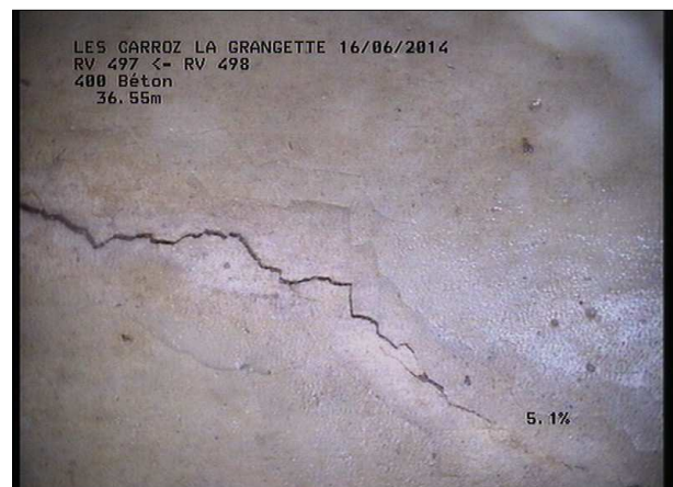
Photo: 1_14B, MPEG #: 160614_1, 00:08:09 36,55m, Fissure transversale (circulaire)
