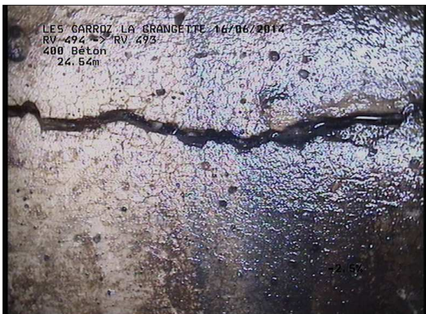
Photo: 7_8B, MPEG #: 160614_1, 00:05:23 24,54m, Fissure transversale (circulaire)
