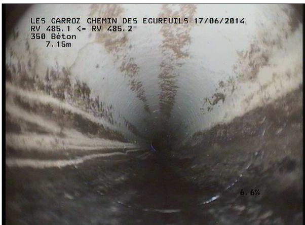
Photo: 18_4A, MPEG #: 160614_1, 00:01:40 7,39m, Fissure transversale (circulaire)
