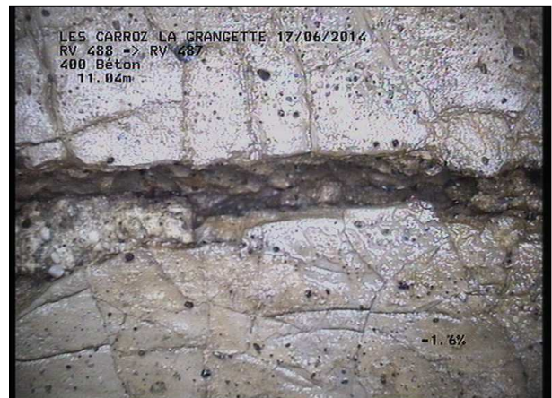
Photo: 13_5B, MPEG #: 160614_1, 00:02:04 11,04m, Fissure transversale (circulaire)
