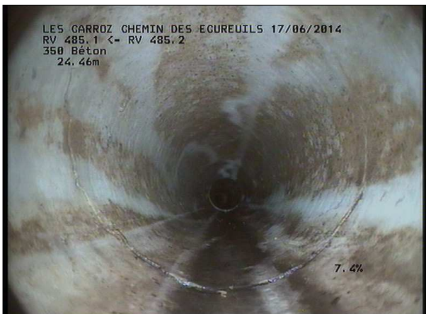
Photo: 18_8A, MPEG #: 160614_1, 00:04:08 24,73m, Fissure transversale (circulaire)
