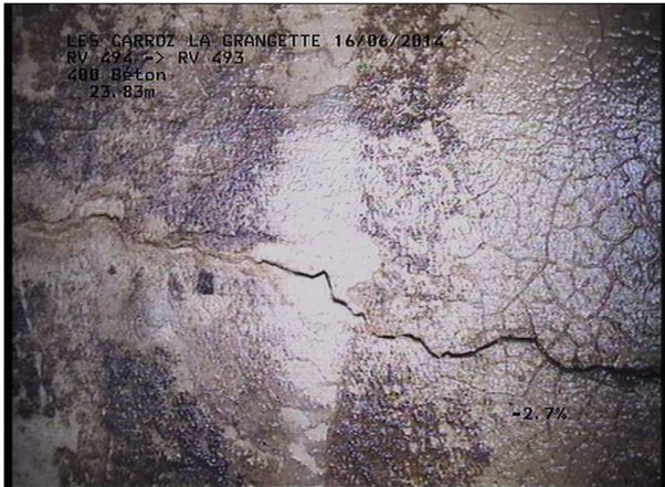
Photo: 7_7B, MPEG #: 160614_1, 00:05:00 23,83m, Fissure transversale (circulaire)
