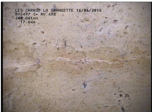
Photo: 1_9B, MPEG #: 160614_1, 00:04:21 17,64m, Fissure transversale (circulaire)
