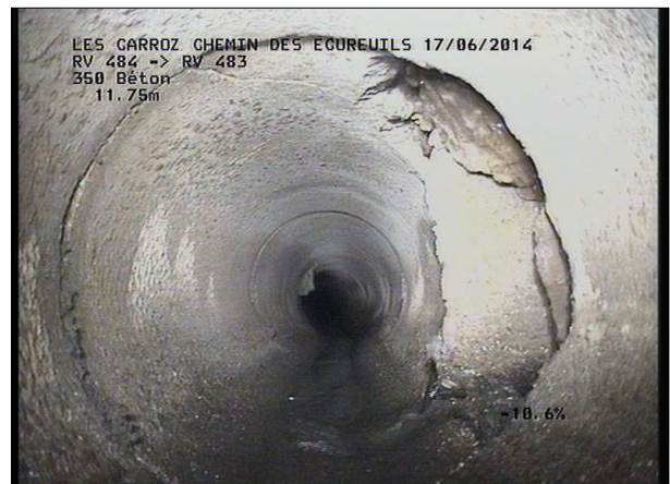
Photo: 21_2A, MPEG #: 160614_1, 00:01:55 12,51m, Interruption de l'inspection franchissement raccordement impossible
