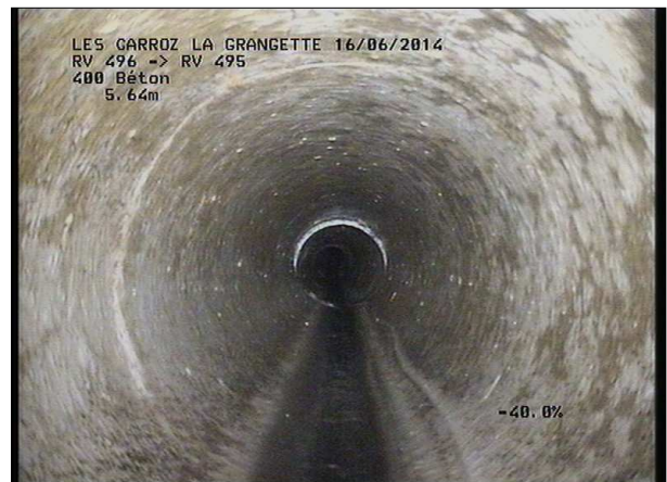
Photo: 5_3A, MPEG #: 160614_1, 00:00:51 6,1m, Fissure transversale (circulaire)
