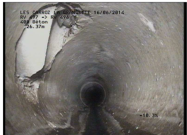
Photo: 4_11A, MPEG #: 160614_1, 00:06:21 27,02m, Raccordement direct à 11 h.
