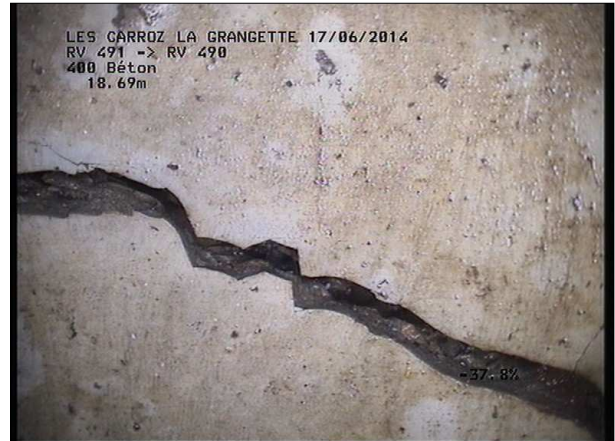
Photo: 10_12B, MPEG #: 160614_1, 00:05:30 18,69m, Fissure transversale (circulaire)
