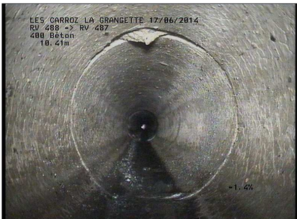
Photo: 13_5A, MPEG #: 160614_1, 00:02:04 11,04m, Fissure transversale (circulaire)
