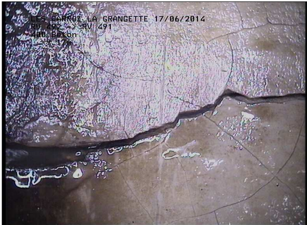
Photo: 9_3B, MPEG #: 160614_1, 00:00:57 9,17m, Fissure transversale (circulaire)
