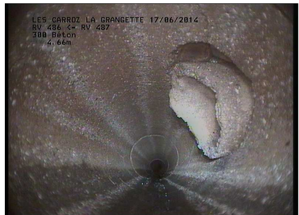
Photo: 15_3A, MPEG #: 160614_1, 00:00:36 4,95m, Raccordement direct à 02 h.
