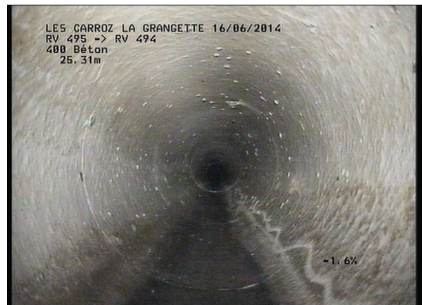
Photo: 6_5A, MPEG #: 160614_1, 00:03:16 25,85m, Fissure transversale (circulaire)
