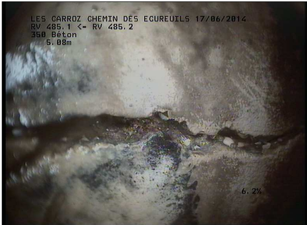
Photo: 18_3B, MPEG #: 160614_1, 00:01:09 5,08m, Fissure transversale (circulaire)
