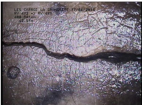
Photo: 9_19B, MPEG #: 160614_1, 00:09:12 42,51m, Fissure transversale (circulaire)
