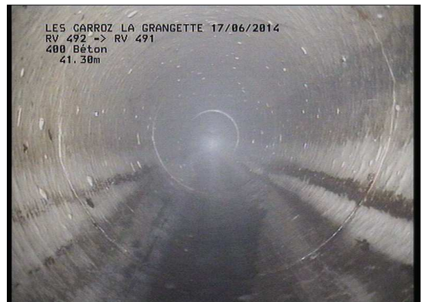
Photo: 9_18A, MPEG #: 160614_1, 00:08:42 41,72m, Fissure transversale (circulaire)
