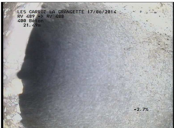
Photo: 12_8B, MPEG #: 160614_1, 00:04:31 21,49m, Raccordement direct à 11 h.
