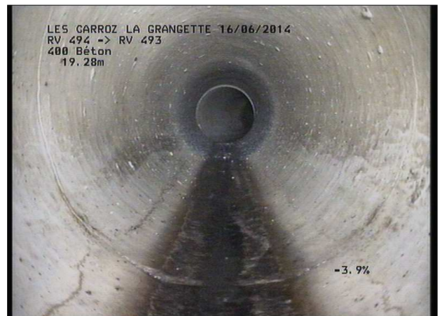
Photo: 7_5A, MPEG #: 160614_1, 00:03:35 19,72m, Fissure transversale (circulaire)
