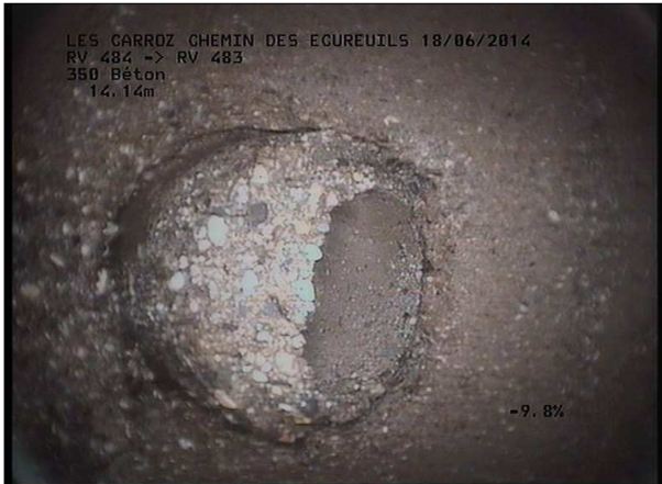
Photo: 23_3B, MPEG #: 160614_1, 00:01:31 14,14m, Raccordement direct à 11 h.
