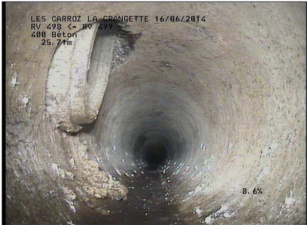
Photo: 2_12A, MPEG #: 160614_1, 00:06:42 26,32m, Raccordement direct à 11 h.
