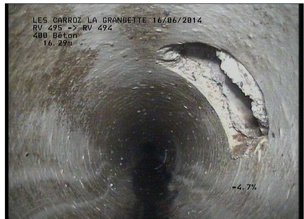
Photo: 6_3A, MPEG #: 160614_1, 00:01:46 16,89m, Raccordement direct à 02 h.
