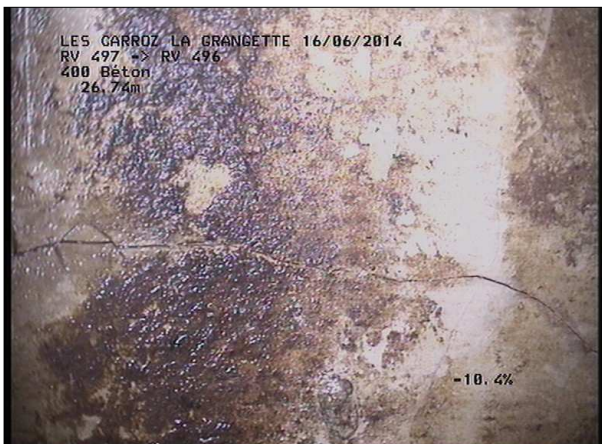
Photo: 4_10B, MPEG #: 160614_1, 00:05:51 26,74m, Fissure transversale (circulaire)
