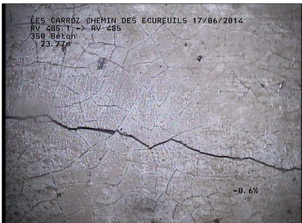
Photo: 19_9B, MPEG #: 160614_1, 00:04:53 23,77m, Fissure transversale (circulaire)
