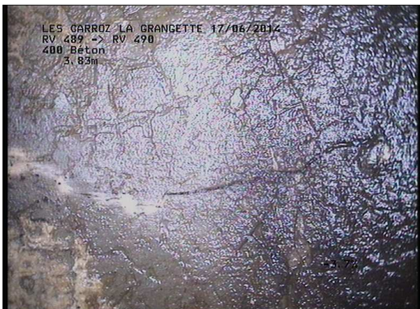
Photo: 11_2B, MPEG #: 160614_1, 00:00:21 3,27m, Fissure transversale (circulaire)
