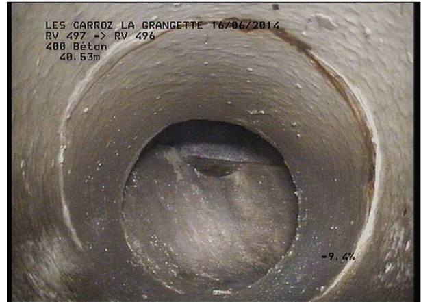
Photo: 4_16A, MPEG #: 160614_1, 00:09:47 40,97m, Fissure transversale (circulaire)
