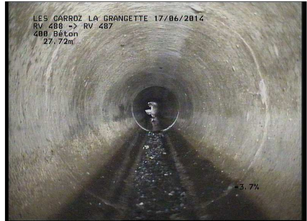
Photo: 13_9A, MPEG #: 160614_1, 00:04:53 28,19m, Fissure transversale (circulaire)
