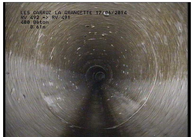
Photo: 9_3A, MPEG #: 160614_1, 00:00:57 9,17m, Fissure transversale (circulaire)
