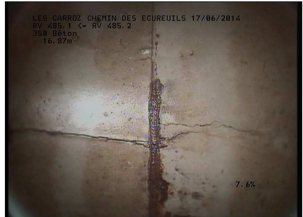
Photo: 18_5B, MPEG #: 160614_1, 00:02:35 16,87m, Armatures visibles à 12 h.
