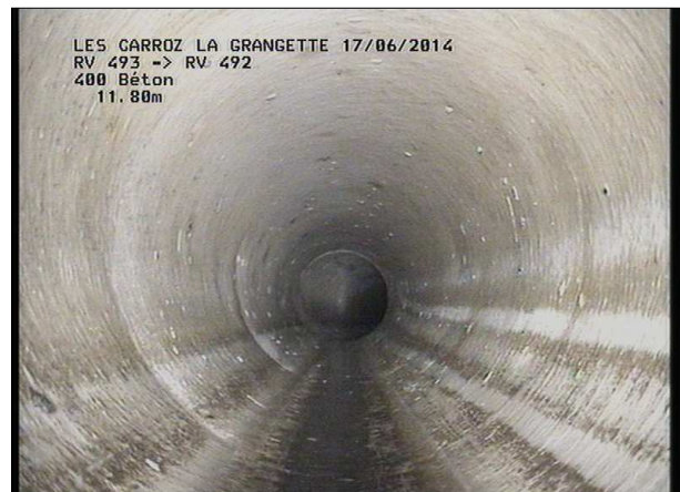
Photo: 8_3A, MPEG #: 160614_1, 00:01:20 12,35m, Fissure transversale (circulaire)
