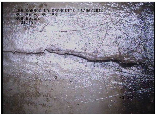
Photo: 6_8B, MPEG #: 160614_1, 00:04:44 31,18m, Fissure transversale (circulaire)
