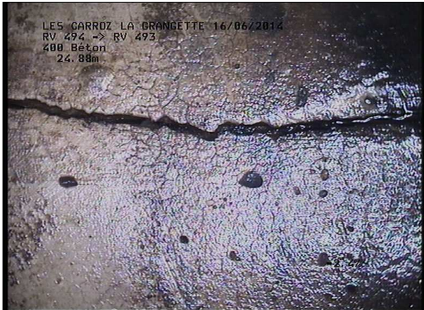
Photo: 7_9B, MPEG #: 160614_1, 00:05:45 24,68m, Fissure transversale (circulaire)
