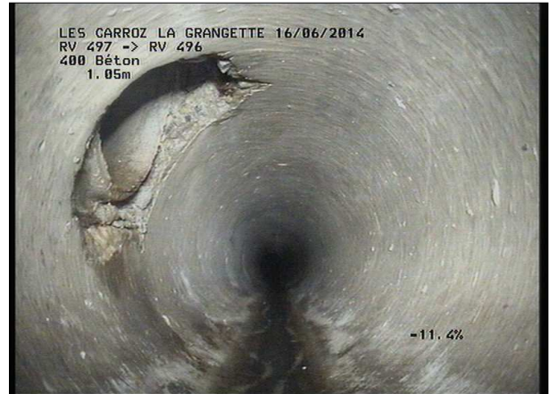
Photo: 4_2A, MPEG #: 160614_1, 00:00:11 1,72m, Raccordement direct à 11 h.
