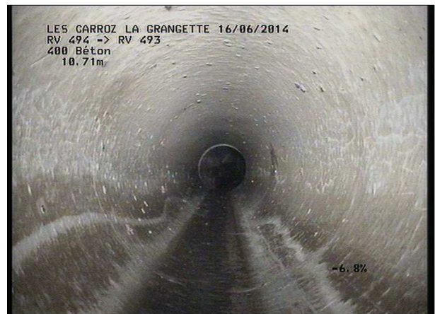
Photo: 7_3A, MPEG #: 160614_1, 00:01:35 11,34m, Fissure transversale (circulaire)
