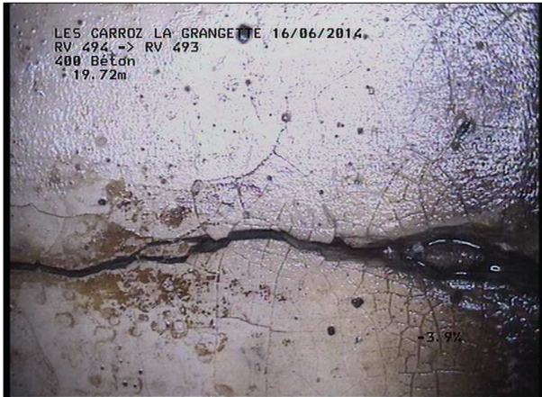
Photo: 7_5B, MPEG #: 160614_1, 00:03:35 19,72m, Fissure transversale (circulaire)
