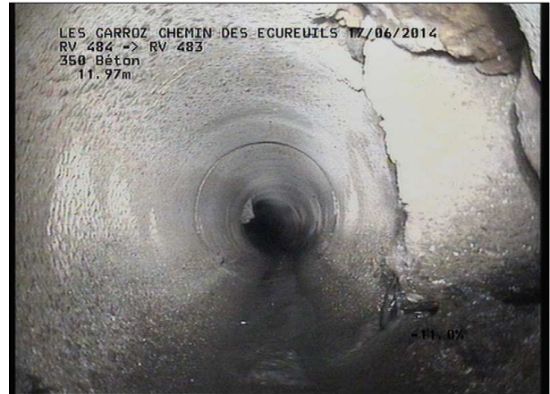
Photo: 21_2A, MPEG #: 160614_1, 00:01:03 12,46m, Raccordement direct à 03 h.
