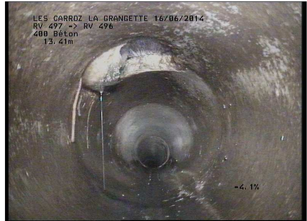
Photo: 4_4A, MPEG #: 160614_1, 00:01:57 14,08m, Raccordement direct à 11 h.
