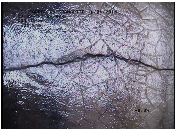
Photo: 6_6B, MPEG #: 160614_1, 00:03:41 26,54m, Fissure transversale (circulaire)
