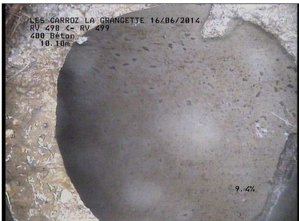
Photo: 2_5B, MPEG #: 160614_1, 00:02:16 10,1m, Raccordement direct à 10 h.
