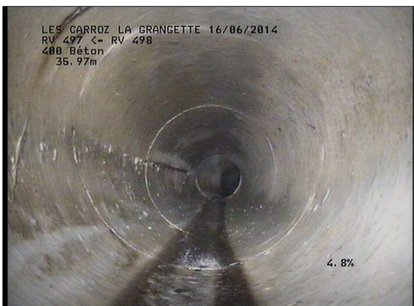
Photo: 1_14A, MPEG #: 160614_1, 00:08:09 36,55m, Fissure transversale (circulaire)
