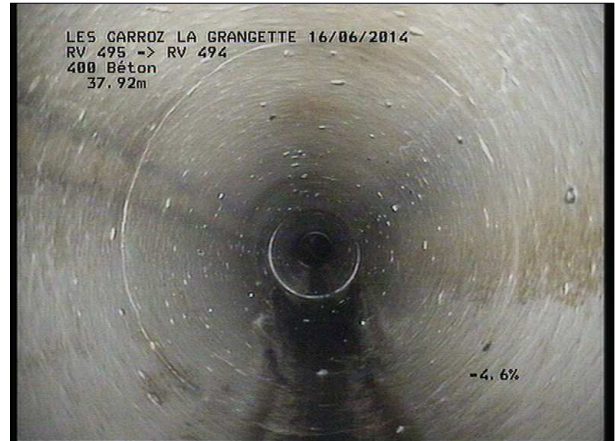
Photo: 6_10A, MPEG #: 160614_1, 00:06:02 38,49m, Fissure transversale (circulaire)
