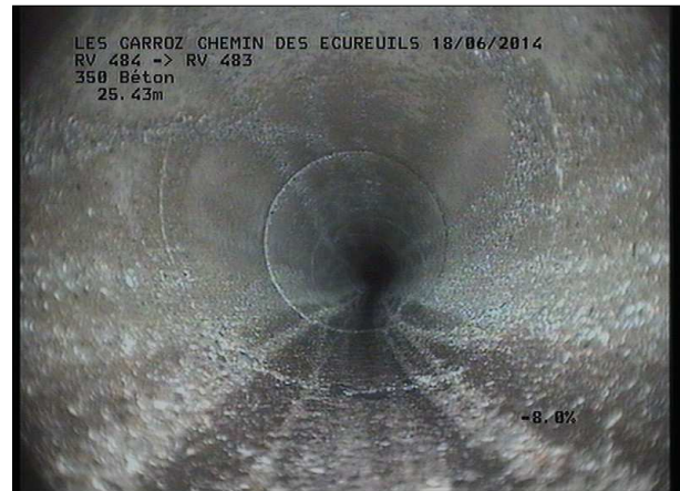
Photo: 23_6A, MPEG #: 160614_1, 00:03:26 25,78m, Fissure transversale (circulaire)
