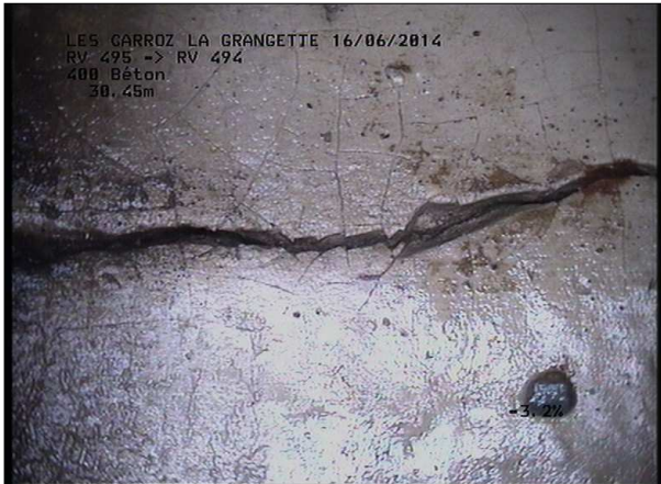
Photo: 6_7B, MPEG #: 160614_1, 00:04:20 30,45m, Fissure transversale (circulaire)
