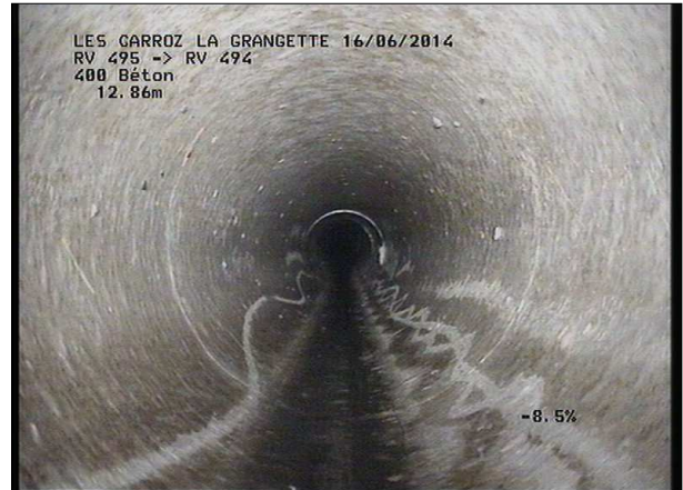
Photo: 6_2A, MPEG #: 160614_1, 00:01:11 13,52m, Fissure transversale (circulaire)
