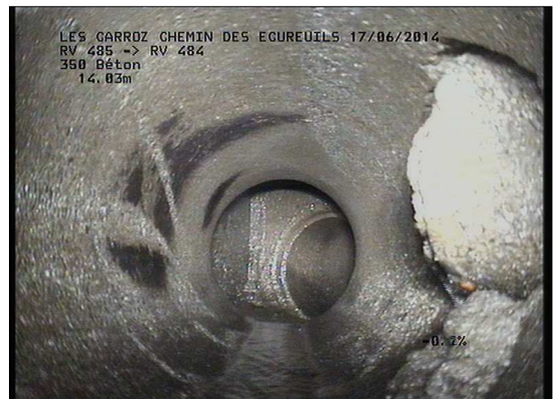
Photo: 20_5A, MPEG #: 160614_1, 00:01:45 14,1m, Raccordement direct à 03 h.
