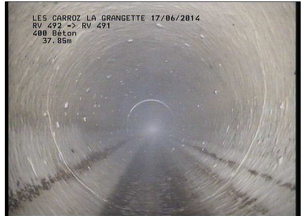
Photo: 9_17A, MPEG #: 160614_1, 00:07:49 38,36m, Fissure transversale (circulaire)
