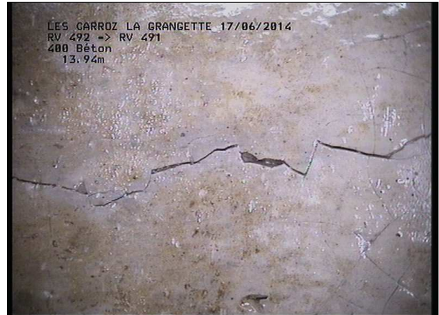
Photo: 9_6A, MPEG #: 160614_1, 00:02:10 13,94m, Fissure transversale (circulaire)
