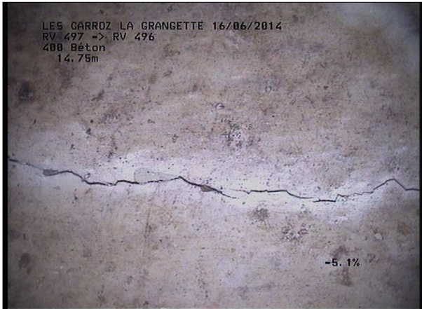
Photo: 4_5B, MPEG #: 160614_1, 00:02:22 14,75m, Fissure transversale (circulaire)
