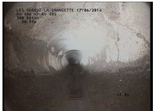
Photo: 16_10A, MPEG #: 160614_1, 00:04:43 30,97m, Fissures multiples de 12 à 12 h.
