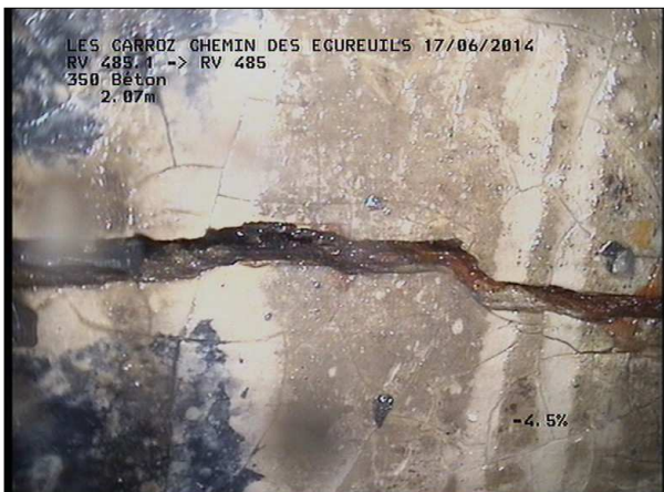
Photo: 19_2B, MPEG #: 160614_1, 00:00:16 2,07m, Fissure transversale (circulaire)
