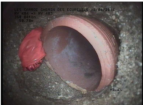
Photo: 23_12B, MPEG #: 160614_1, 00:08:18 50,78m, Raccordement direct à 01 h.
