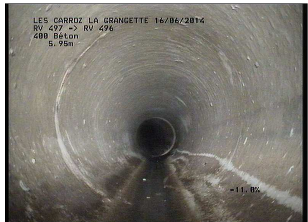
Photo: 4_3A, MPEG #: 160614_1, 00:00:54 5,95m, Fissure transversale (circulaire)
