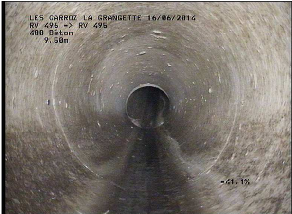
Photo: 5_6A, MPEG #: 160614_1, 00:02:08 10,04m, Fissure transversale (circulaire)
