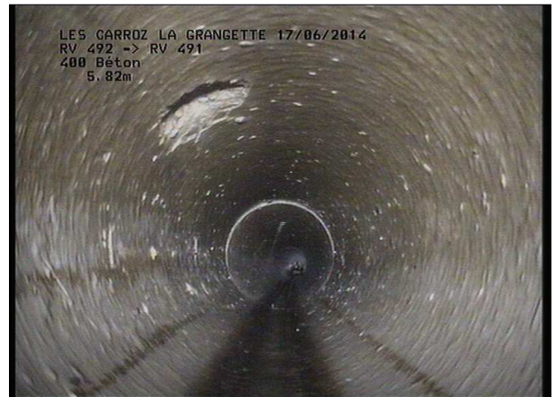
Photo: 9_2A, MPEG #: 160614_1, 00:00:33 6,45m, Perforation à 11 h.
