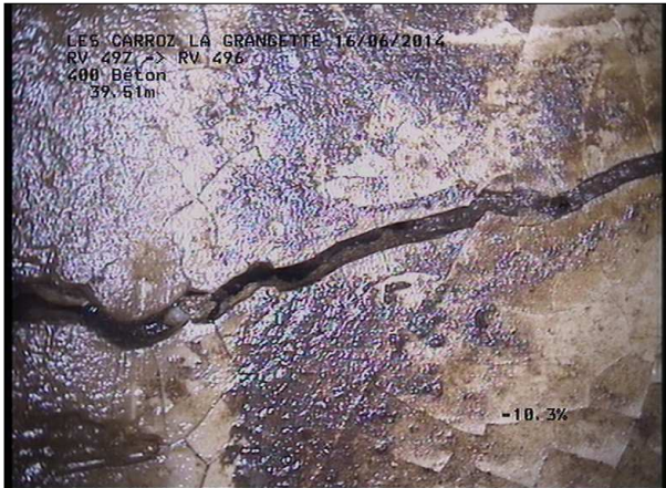
Photo: 4_15B, MPEG #: 160614_1, 00:09:17 39,51m, Fissure transversale (circulaire)
