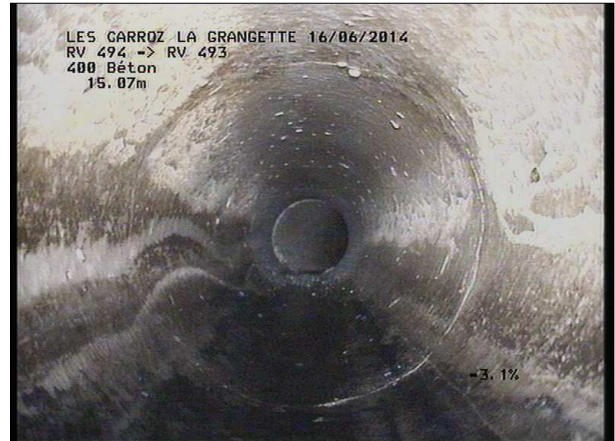
Photo: 7_4A, MPEG #: 160614_1, 00:02:33 15,66m, Fissure transversale (circulaire)
