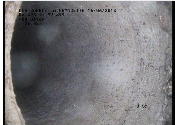
Photo: 2_12B, MPEG #: 160614_1, 00:06:42 26,32m, Raccordement direct à 11 h.
