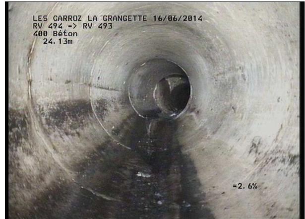
Photo: 7_8A, MPEG #: 160614_1, 00:05:23 24,54m, Fissure transversale (circulaire)
