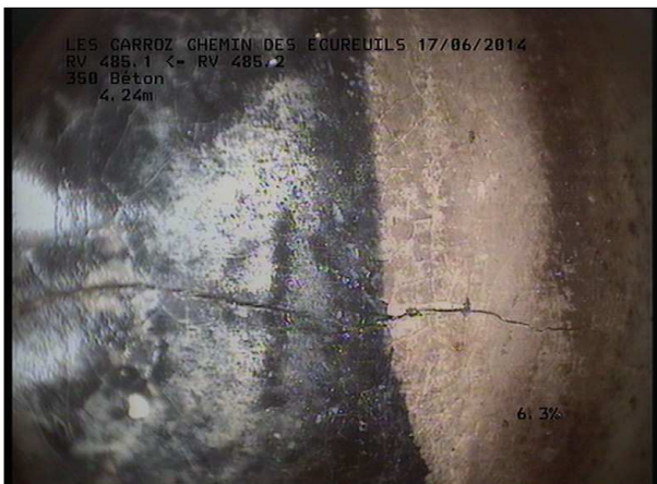
Photo: 18_2B, MPEG #: 160614_1, 00:00:33 4,24m, Fissure transversale (circulaire)
