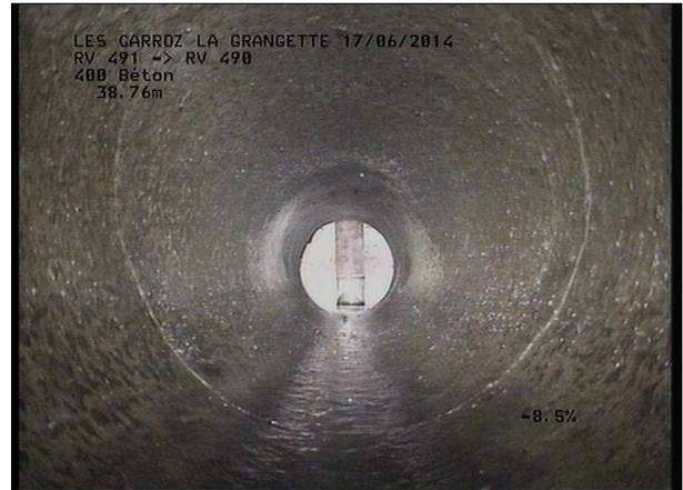
Photo: 10_21A, MPEG #: 160614_1, 00:09:31 39,25m, Fissure transversale (circulaire)
