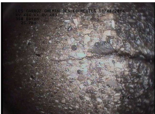
Photo: 23_6B, MPEG #: 160614_1, 00:03:26 25,78m, Fissure transversale (circulaire)
