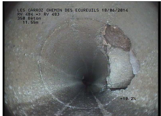
Photo: 23_2A, MPEG #: 160614_1, 00:01:07 12,07m, Raccordement direct à 03 h.
