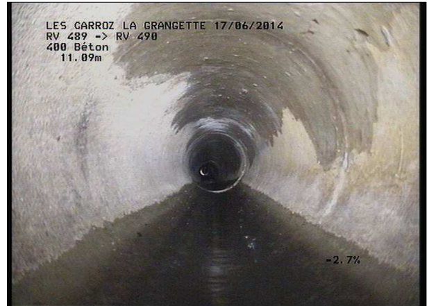
Photo: 11_4A, MPEG #: 160614_1, 00:01:48 11,67m, Fissure transversale (circulaire)
