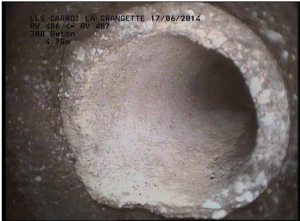
Photo: 15_3B, MPEG #: 160614_1, 00:00:36 4,95m, Raccordement direct à 02 h.
