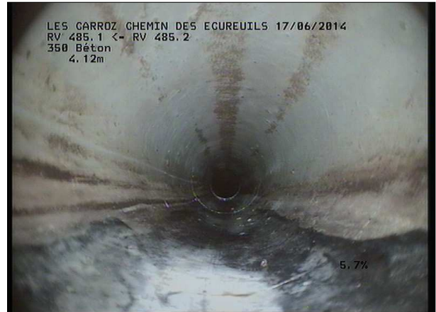
Photo: 18_2A, MPEG #: 160614_1, 00:00:33 4,24m, Fissure transversale (circulaire)
