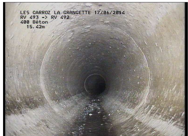
Photo: 8_5A, MPEG #: 160614_1, 00:02:13 16,04m, Fissure transversale (circulaire)
