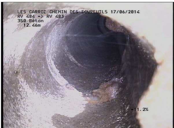
Photo: 21_2B, MPEG #: 160614_1, 00:01:03 12,46m, Raccordement direct à 03 h.
