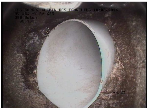
Photo: 23_8B, MPEG #: 160614_1, 00:05:02 38,13m, Raccordement direct à 01 h.
