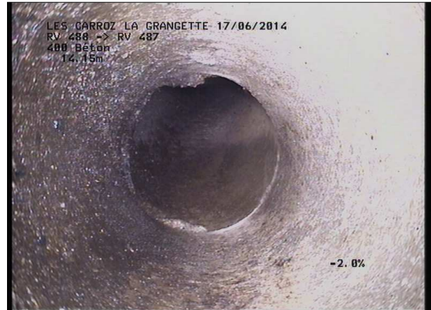
Photo: 13_6B, MPEG #: 160614_1, 00:02:38 14,15m, Raccordement direct à 10 h.
