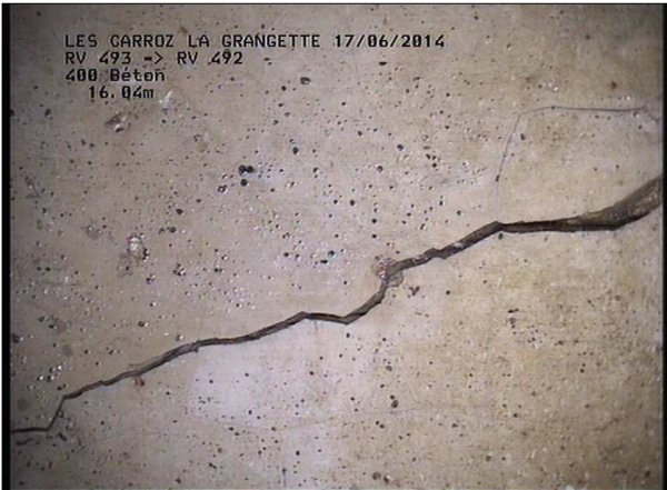
Photo: 8_5B, MPEG #: 160614_1, 00:02:13 16,04m, Fissure transversale (circulaire)
