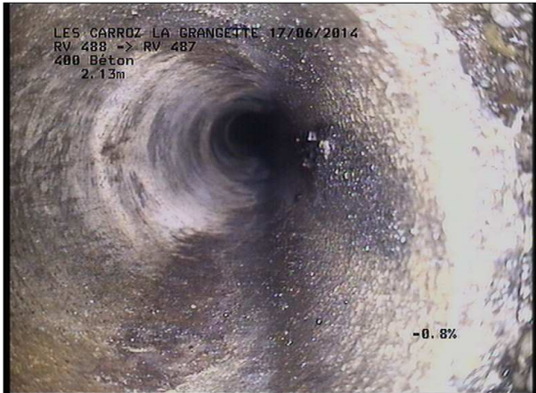
Photo: 13_3B, MPEG #: 160614_1, 00:00:30 2,13m, Raccordement direct à 03 h.
