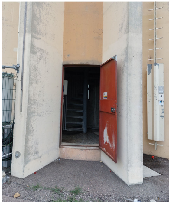
FIGURE 24 – ENTREE DU RESERVOIR DE COLOMBIER
