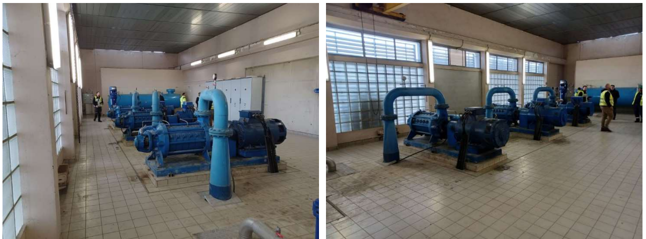
Figure 152 - Pompes de la station de surpression
