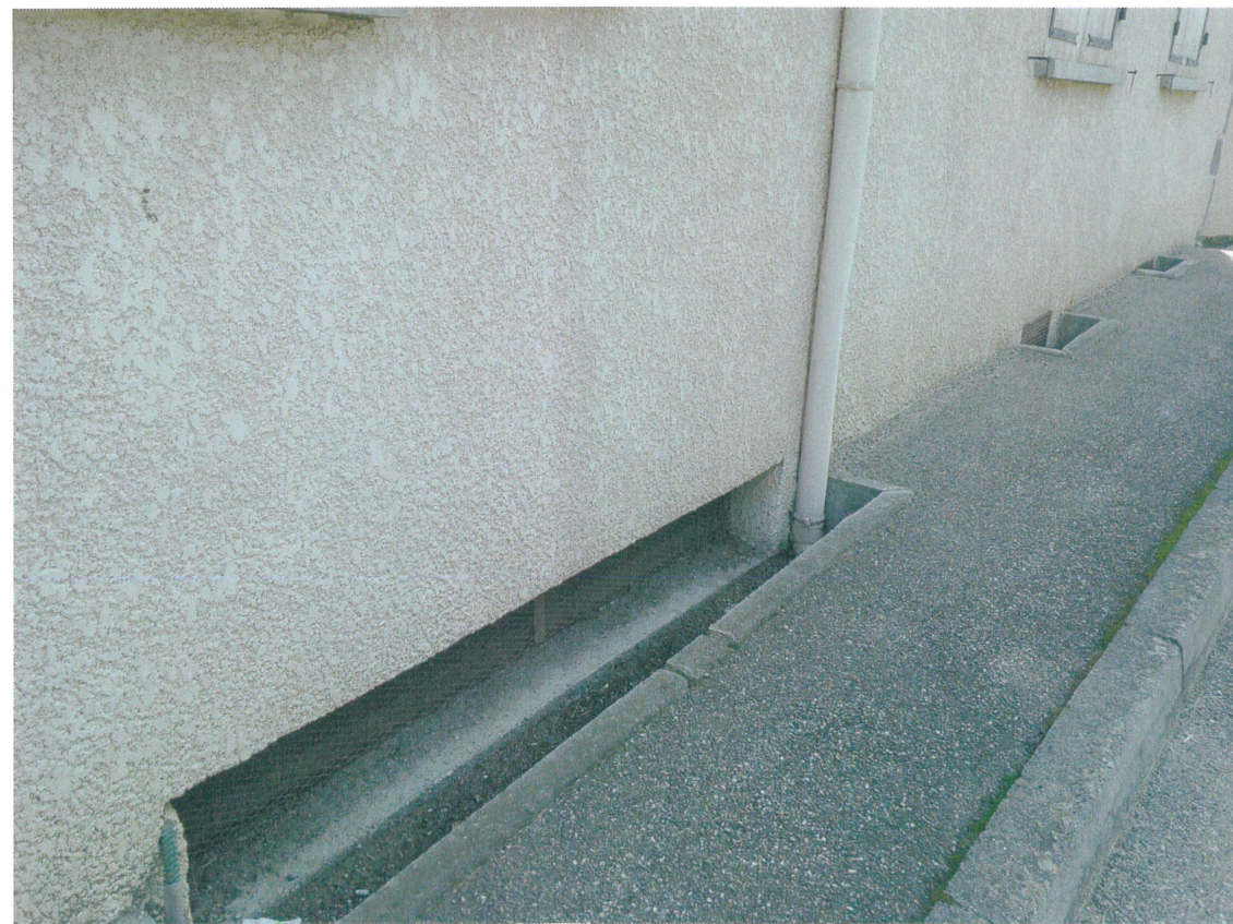
F3 - Inondation de caves (CHAG-D2)
