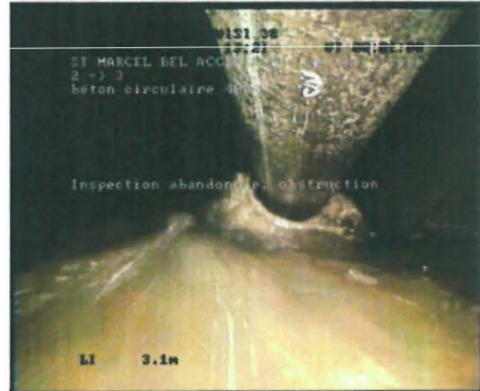
Photo: 0000016.JPG, 00:00:59 3,12m, Inspection abandonnée, obstruction
