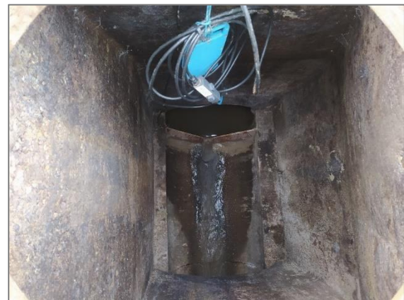
Figure 54 : Installation PDM Garanche Bourg
