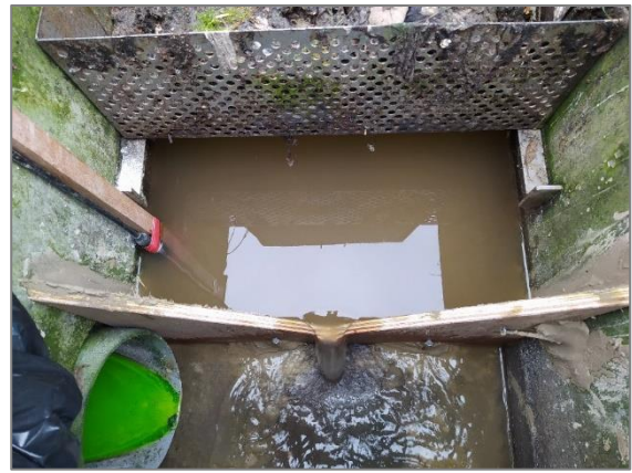
Figure 60 : Installation PDM Mont Brouilly STEP
