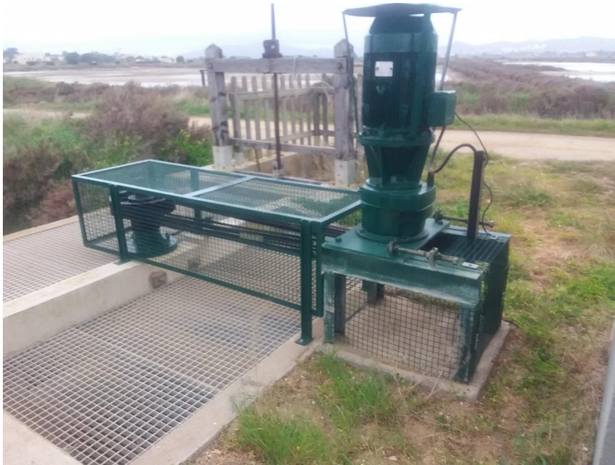
FIGURE 79 – STATION DE POMPAGE LIANT DIFFERENTS CANAUX D'IRRIGATION
