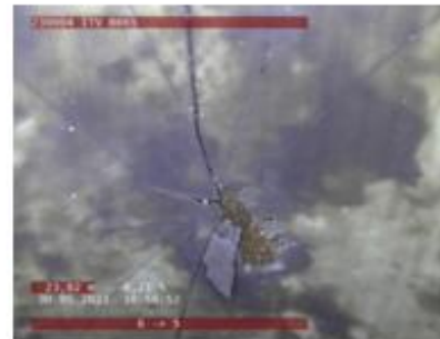
D : Rupture + Fissure complexe
